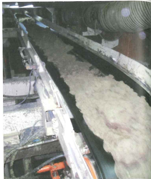
Above: Figure 1, the conveyor carries the conditioned soil from the TBM face; Below: Figure 2, a graph to indicate the volume of grout injected as the tunnel advances by rings
