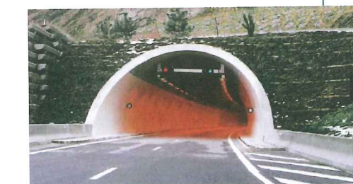
Below: Counterbeam lighting at the Aiguebelle Tunnel portal in southeast France using Schreder FR4 luminaires with 400W HPS lamps
