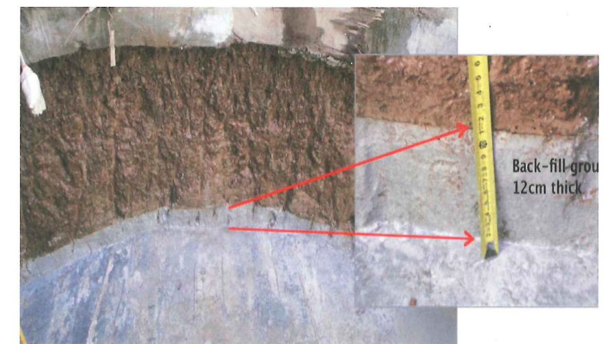
Above: Figure 3, a clear view of the backfill used to fill the annular space left between the ground and the tunnel lining as the TBM advances
