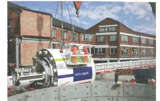
Right: Preparing to lower Herrenknecht TBM 'Cleopatra' down the Eade Road shaft.
