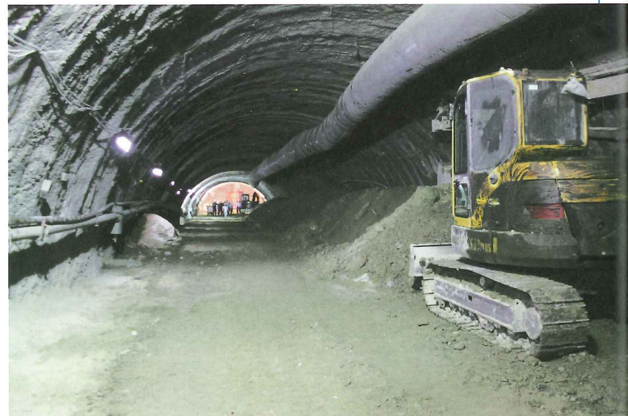
Above: Metro makes the first link in the tunnel excavation for the expansion of Line 5-Lilac. The connection is near a service pit
