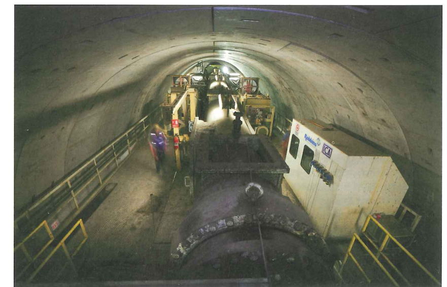
Above: The 10.2 m diameter Robbins EPB is the largest TBM ever to bore in Mexico
