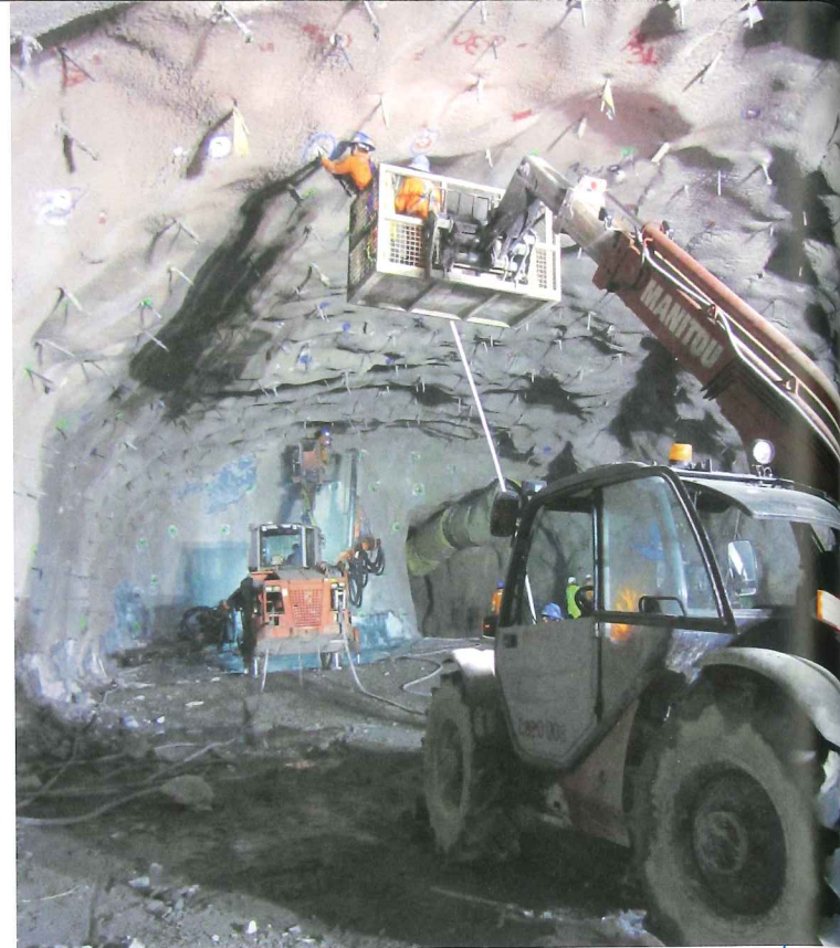
Right: Excavation through grandiorite for the crown of the powerhouse complex, which has an overburden of some 750m and requires 25,000m 3 of rock to be removed
