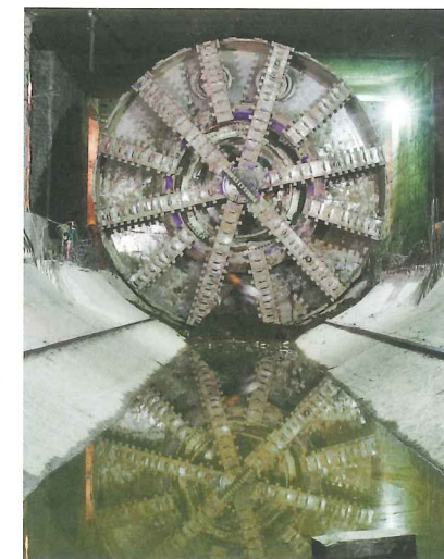
Above: Despite numerous planned stoppages through each station site, the Robbins EPBM achieved rates of up to 135m in a week, and managed 400m per month on average
