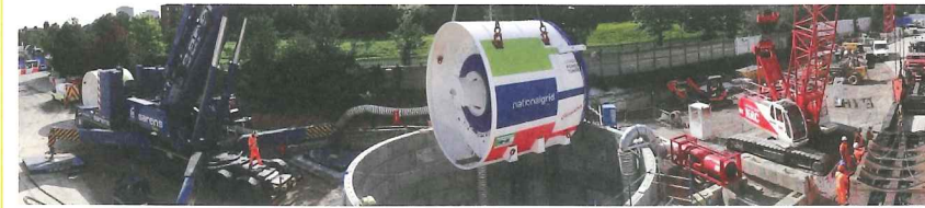
Above: Starting to lower Herrenknecht TBM 'Cleopatra' down the Eade Road shaft (looking South) using a 800t mobile crane
