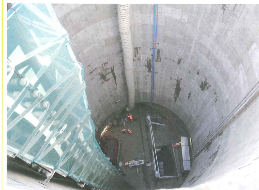
Above: View down the Eade Road shaft showing muck car tippler device, spoil hopper, and the net-enclosed vertical spoil conveyor
