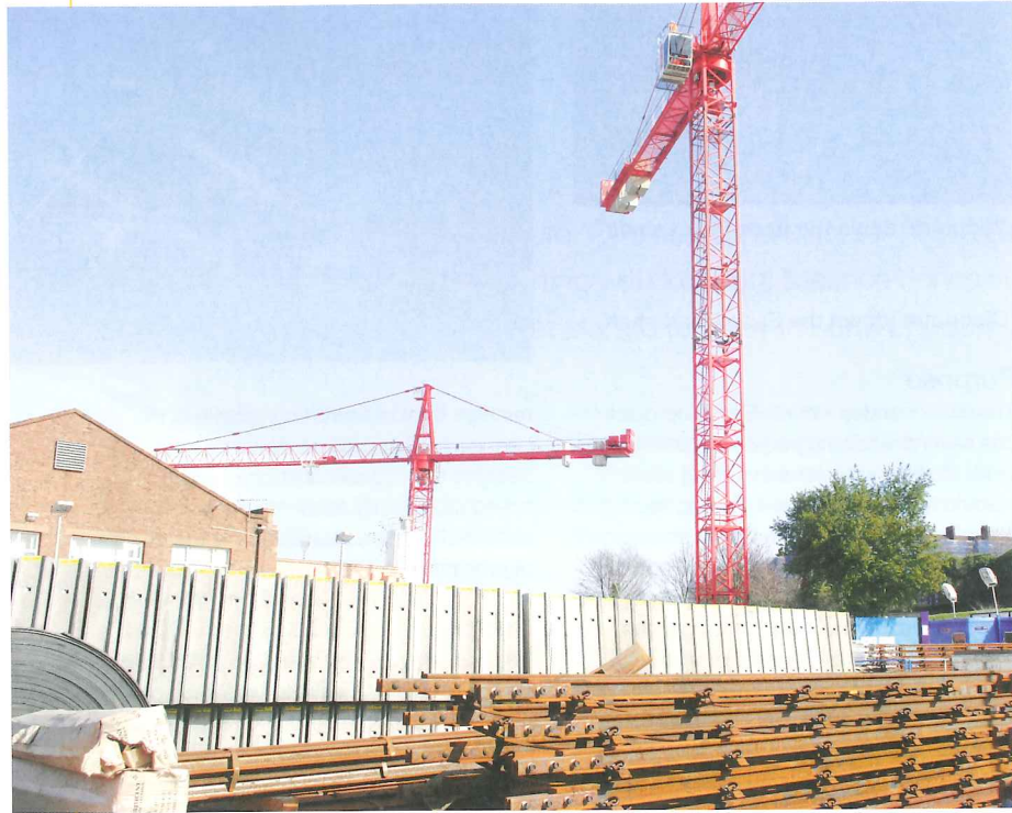
Left: Both Eade Road tower cranes seen from the main materials storage area
