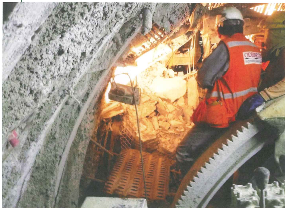
Left: The 1.5km deep Olmas Trans-Andean tunnel is being cut through sever squeezing ground
