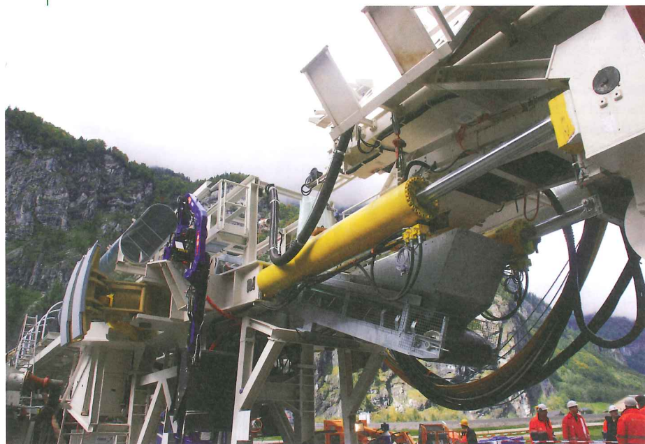
Above: Overhead belt conveyor for spoil through the Linthal back-up system (Photo: Rowa Tunnel Logistics)
