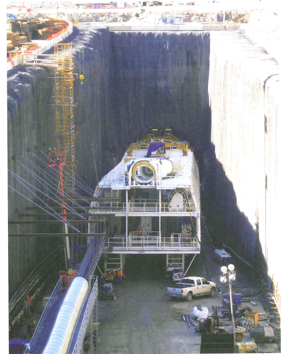
Above: The three-deck Rowa back-up for the Robbins 'Big Becky' TBM on the new Niagara project. Note belt conveyor and ventilation duct
