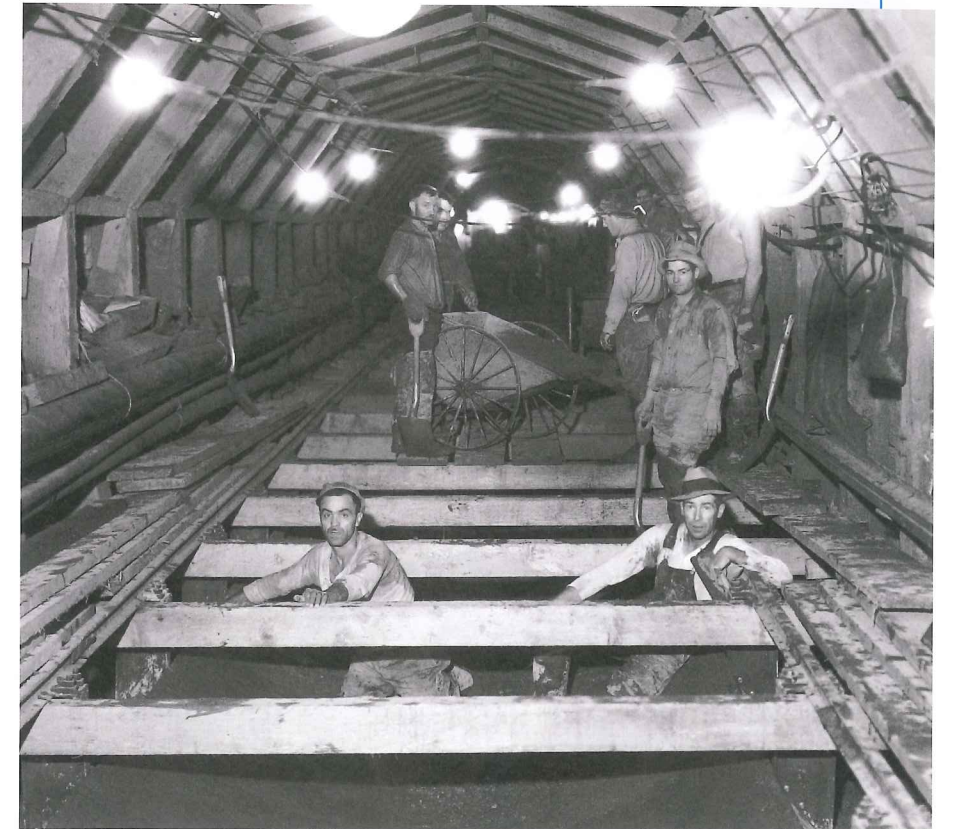
Above: Construction work on the original Irvington tunnel in 1931. © San Francisco Public Utilities Commission; Horace Chaffee
