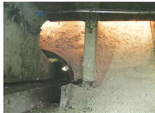
Above: The foot of the jacked deck rested on a slide track. As the structure advances, the crown and side of the tunnel is broken out to reveal the track; Below left: Visible section of tunnel, deck foot and slide track as T&T visits
