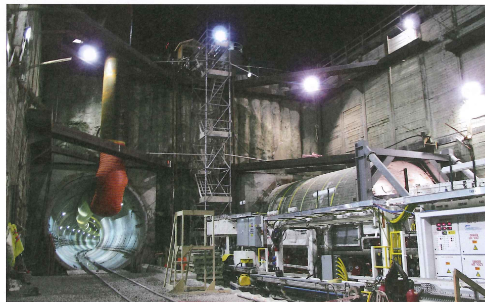
Above: Moley follows sister TBM Holey to excavate Toronto's Spadina subway extension
