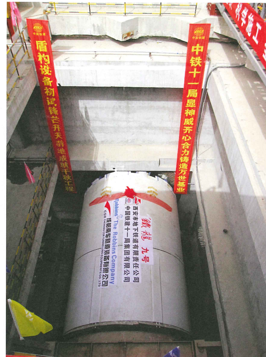
Above: The first of two Robbins EPBMs was launched on Lot 12 of the Xi'an metro in June 2010, and is now currently on its last section of tunnel. (See article on page 32)
