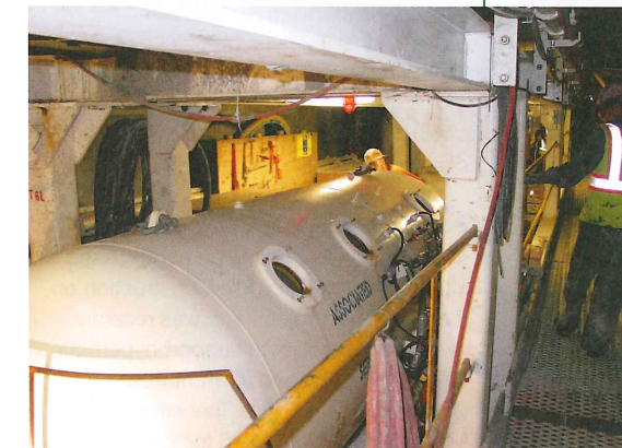
Above: The DART (Diver Attendant Recompression Transportable) chamber arrives at the TBM back-up on the Brightwater project (Photo: Edmond Kay); Below left: Inside a 1.8m-diameter decompression airlock equipped for oxygen breathing (Photo: Specialist Plant)
