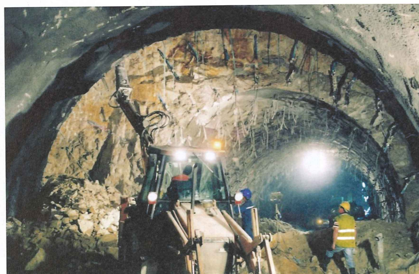
Above: Excavating a tunnel previously strengthened with Sireg Durglass continuous glass-fibre and polymer elements including grouting tubes
