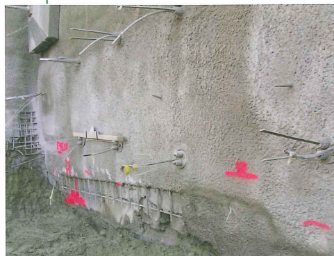
Below: Use of Sireg glass-fibre and polymer elements, including a grouting tube, in anchors installed in a tunnel portal face. Below right: Using jet grouting semi-horizontally, as developed by Rocksoil, to form a canopy around the excavated tunnel using a special rig
