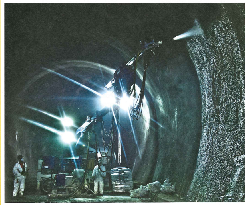
Left: Applying BASF Meyco Masterseal in Hindhead Tunnel using standard robotic spraying equipment
