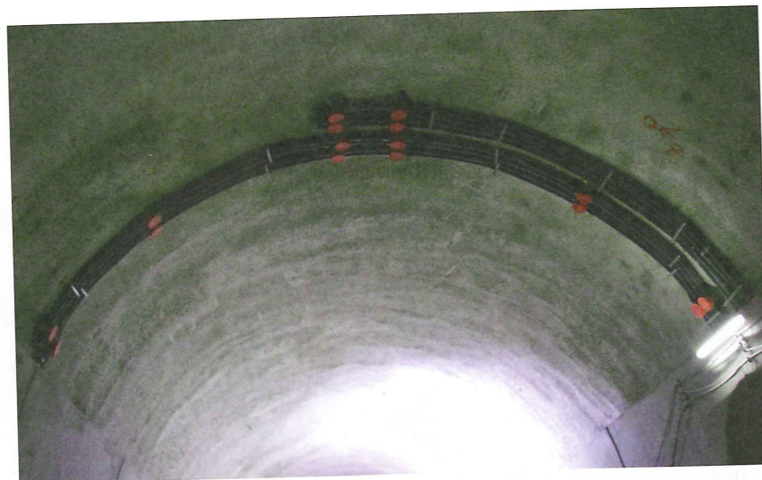
Above: Other membrane penetrations such as duct fixings may require non-corroding fixings and hand-applied sealing
