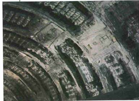
Above: Major fire damage to the concrete lining of the running tunnel with spalling from and behind the steel reinforcement
