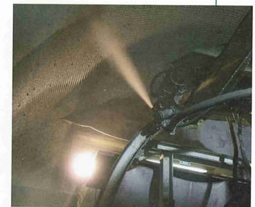
Above: Spraying Fireshield through and onto the stainless steel mesh by remote spraying unit
