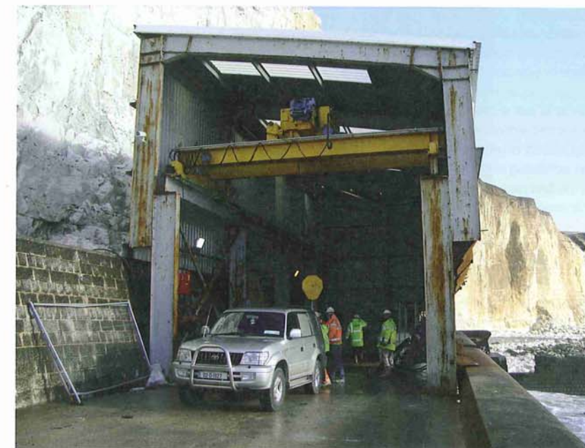
Above: The promenade shaft awaiting arrival of the TBM, exposed to the elements at the bottom of the cliffs
