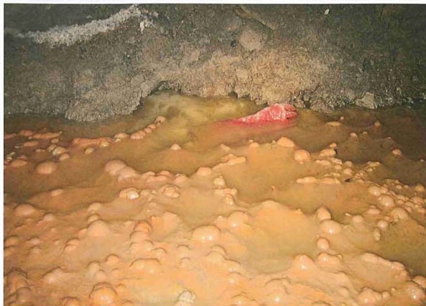
Above: Glycol de-icer created an ideal environment for concrete-eating microbes at the Helsinki airport link project
