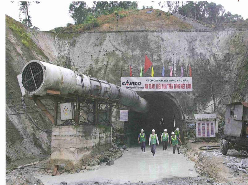
Above: Excavation on the A Luoi hydropower project will be completed in April
