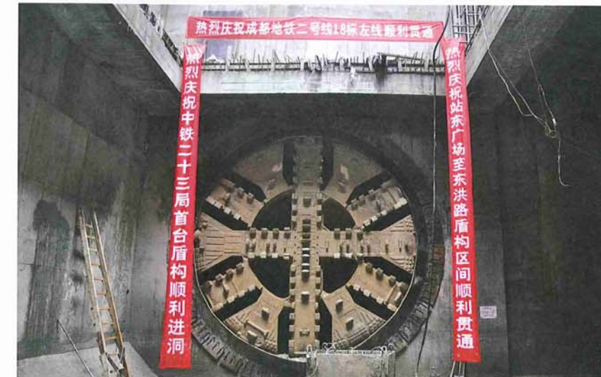
Above: The 6.3m diameter EPB at China's Chengdu Metro Line 2 achieved a project record of 180m in one week while excavating through the area's permeable alluvium
