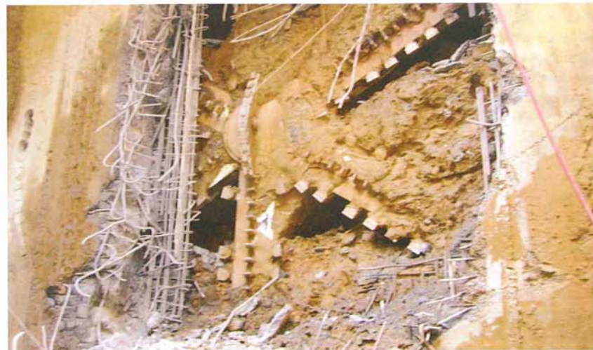
Above: New Delhi Breakthrough: Rapidly expanding population and lack of infrastructure make urban rail tunnels, such as the New Delhi Metro project, of paramount importance
