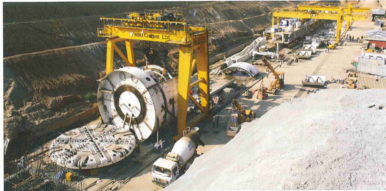
Above: Sleemanabad Onsite Assembly: India has much tunneling potential, particularly for urban rail tunnels, hydroelectric tunnels, and water transfer tunnels like the Sleemanabad Tunnel Project
