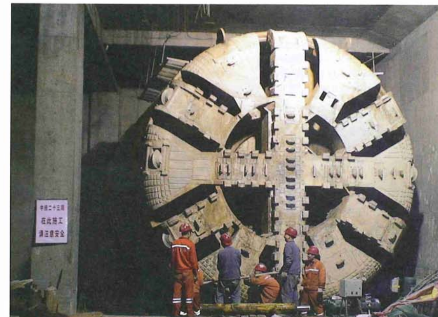
Below: The Robbins EPB at Chengdu Metro excavated an area of harder ground and glacial boulders below a river, requiring only three cutter changes. The machine broke through in December 2010
