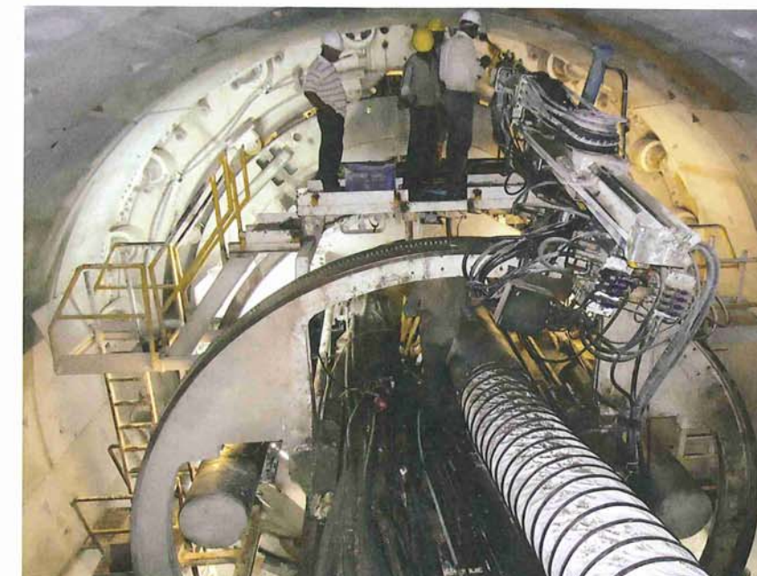
Above: Probe Drilling at Veligonda: Probe drilling operations on a 10m Double Shield TBM for the Veligonda Water Transfer Tunnel in arid Andhra Pradesh state
