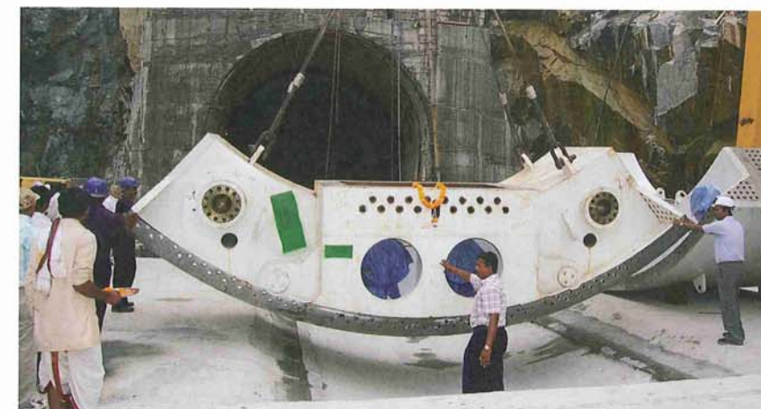
Above: AMR Onsite Assembly: India's water transfer projects, such as the AMR tunnels, have the potential to harness the country's floodwaters from seasonal monsoons for irrigation and drinking water
