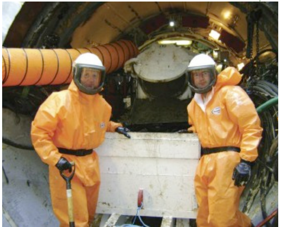
Above: Full personal protective equipment including a respiratory helmet is necessary in dealing with contaminated ground, as here at West Ham, east London [Photo: Costain]
