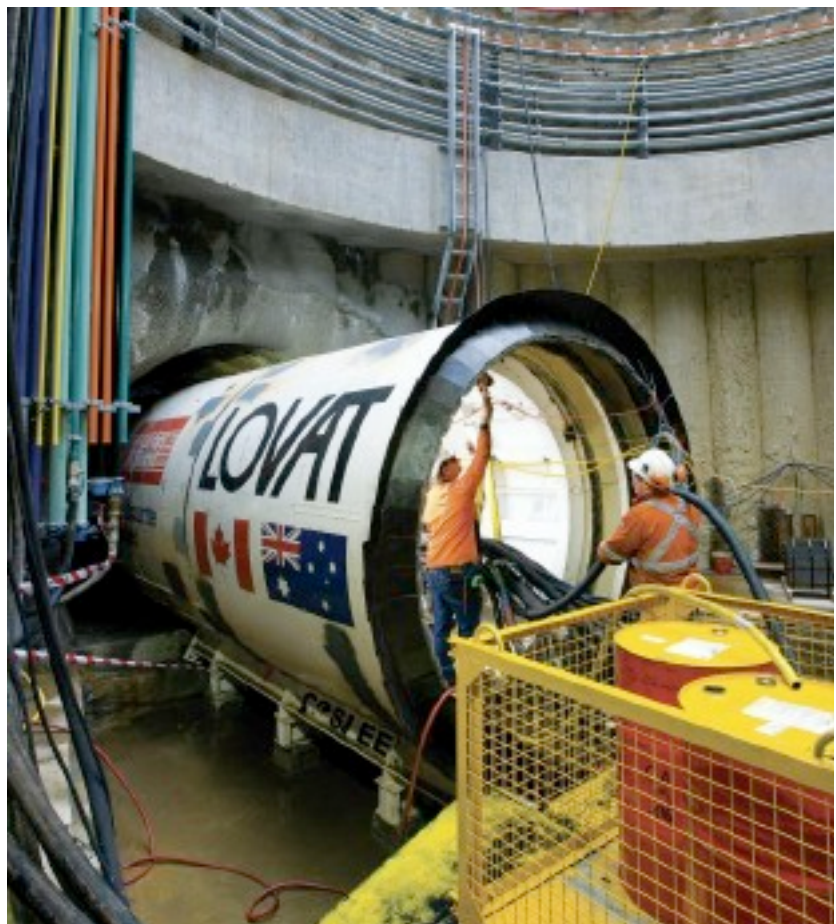
Above: A Lovat EPB TBM used for the Main Sewer Replacement Project in Melbourne
