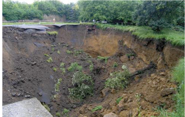
Above: Surface situation at the time of the collapse in the north tube of the Blanka Tunnel
