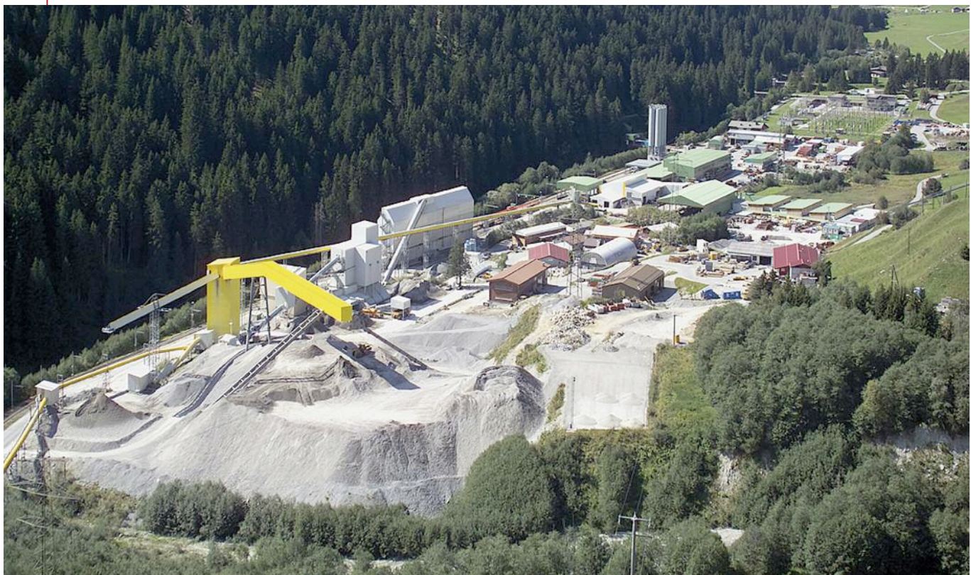
Below: The Sedrun workcamp is sited outside the portal for the shaft tunnel in a small valley 150m below the village. A small rack and pinion railway was built to carry materials in and spoil is removed by conveyor. Picture Alptransit Gotthard
