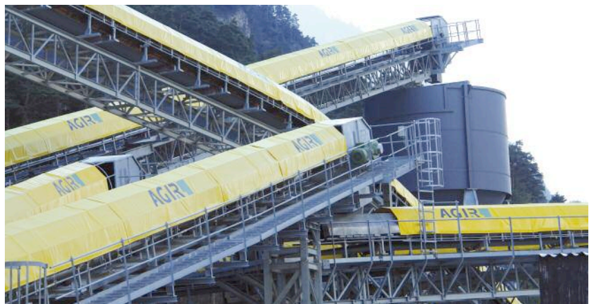
Above, top: Testing the piora: a special exploratory drive driven at an angel from Faido was made to a level 300m above the main tunnel line cores were made from the end Above, bottom: Spoil handling conveyors for the batching plants at the Erstfeld portal site. Picture courtesy of AlpTransit Gotthard
