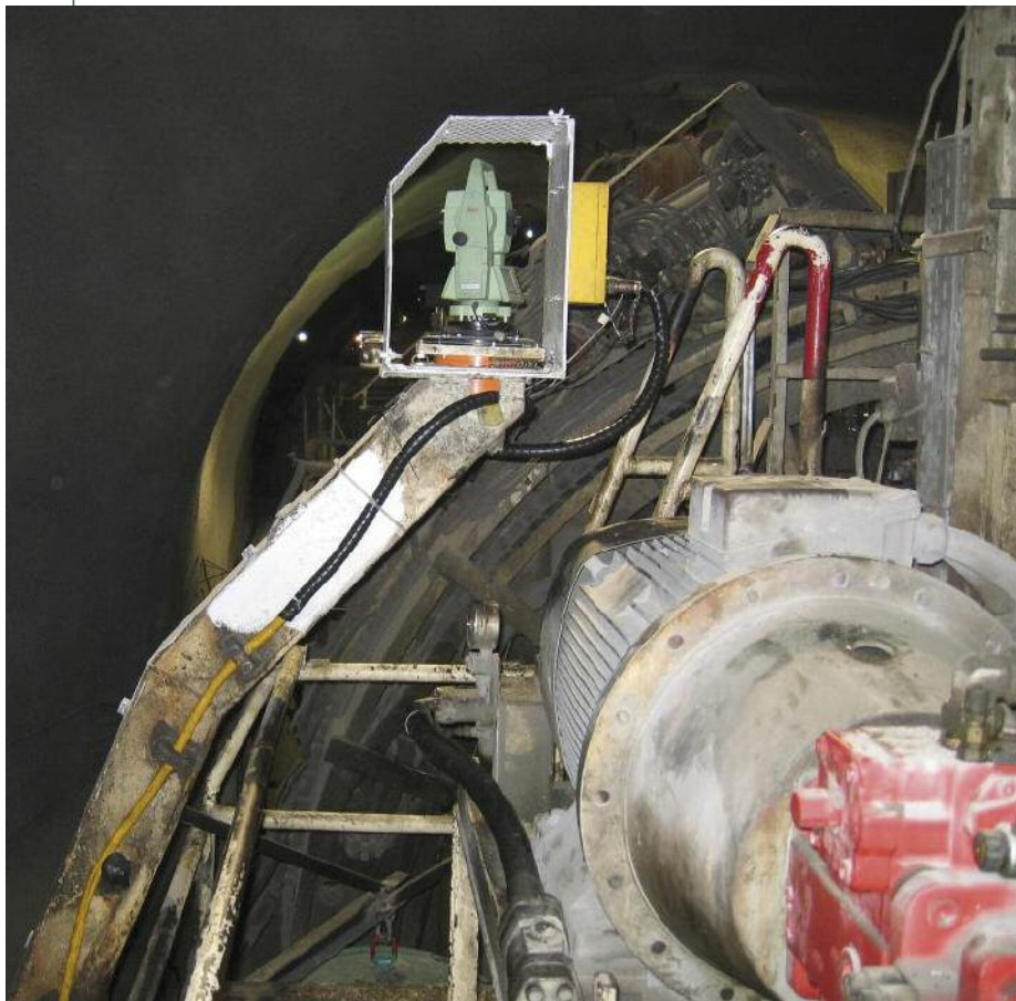
Left, top: Fig. 5 – Divert frame with machine station;
