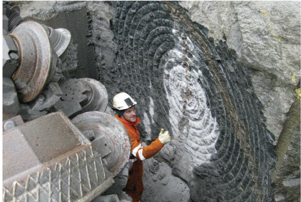
Above: A worker okays checks the tunnel face on the Eysturoy Island project
