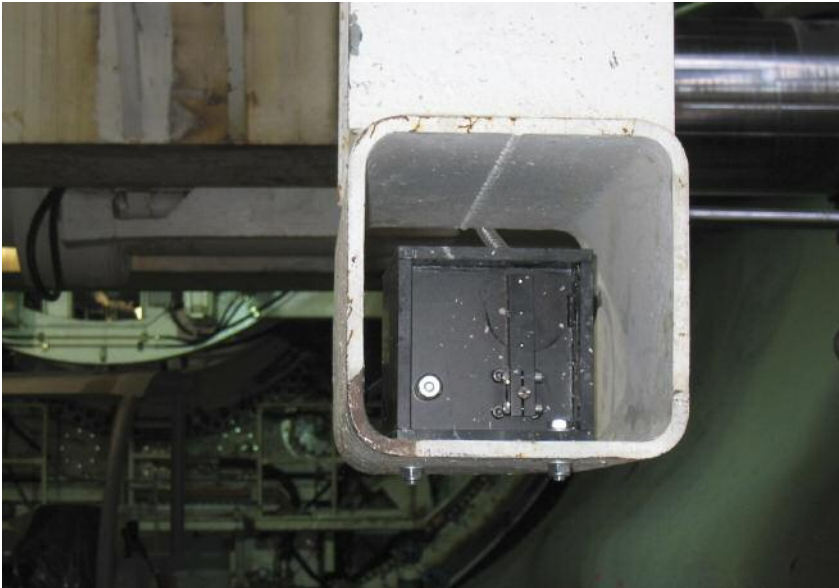
Left, top: Fig. 2 – Installed shutter prisms (closed)
