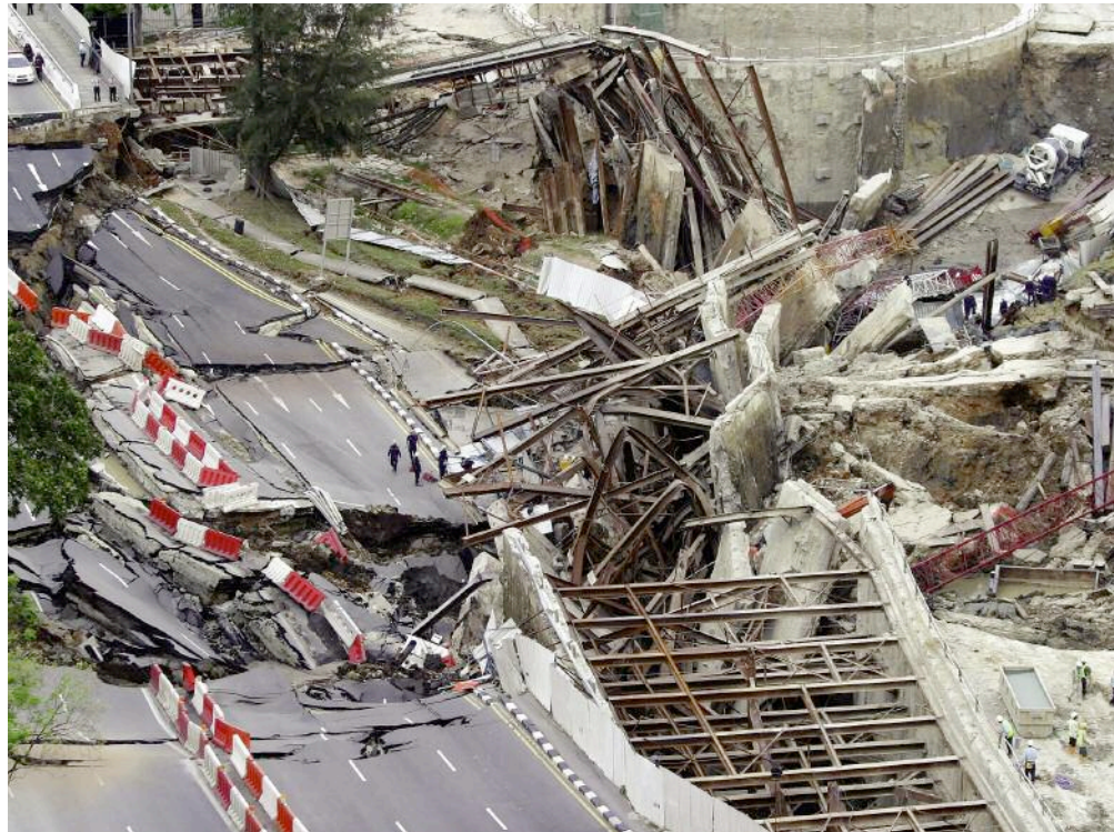
Above: The Nicoll Highway collapse in 2004
