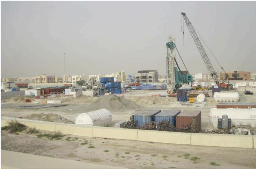
Left: The 6.3m diameter TBM is set to arrive and be installed at the launch shaft in October
