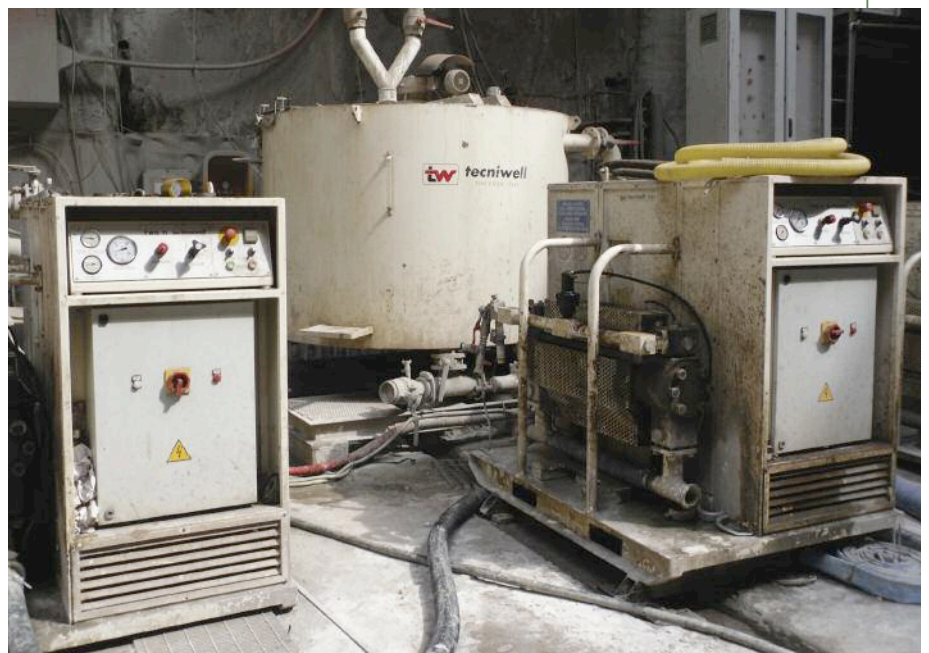
Right: Final tank where the Component A is stocked and then pumped to the tunnels
