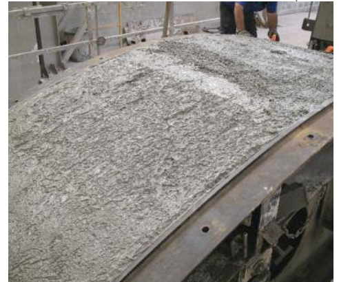
Above: Forming pre-cast segments using EPC BarChip macrosynthetic fibre-reinforced concrete for a tunnel in Malaga, Spain
