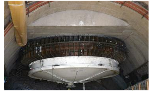
Above: The TBM's cap and the 2-seal ring as it enters the shaft
