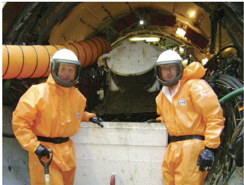
Below: Contamination at Shaft T1 required shaft sink to be adapted
