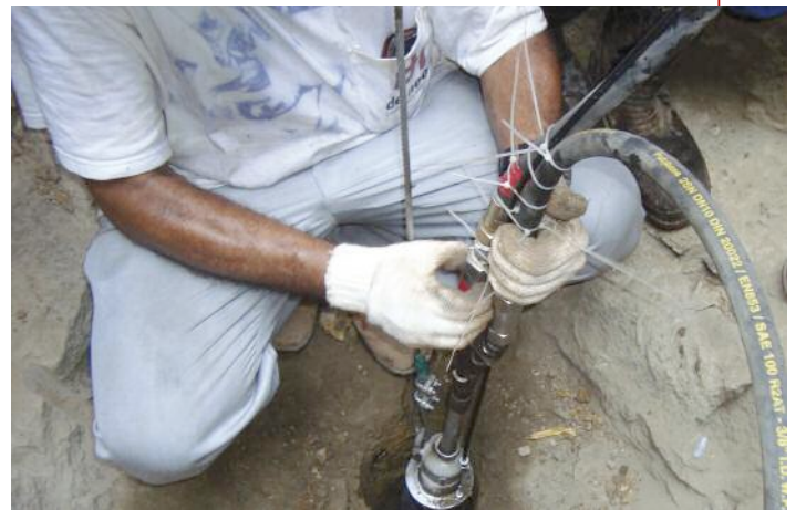
Top: Tunnel damage repair included a stainless-steel plate Above: Preparing to inject 2-part PU grout into the borehole Bottom left: The borehole grout reached the tunnel
