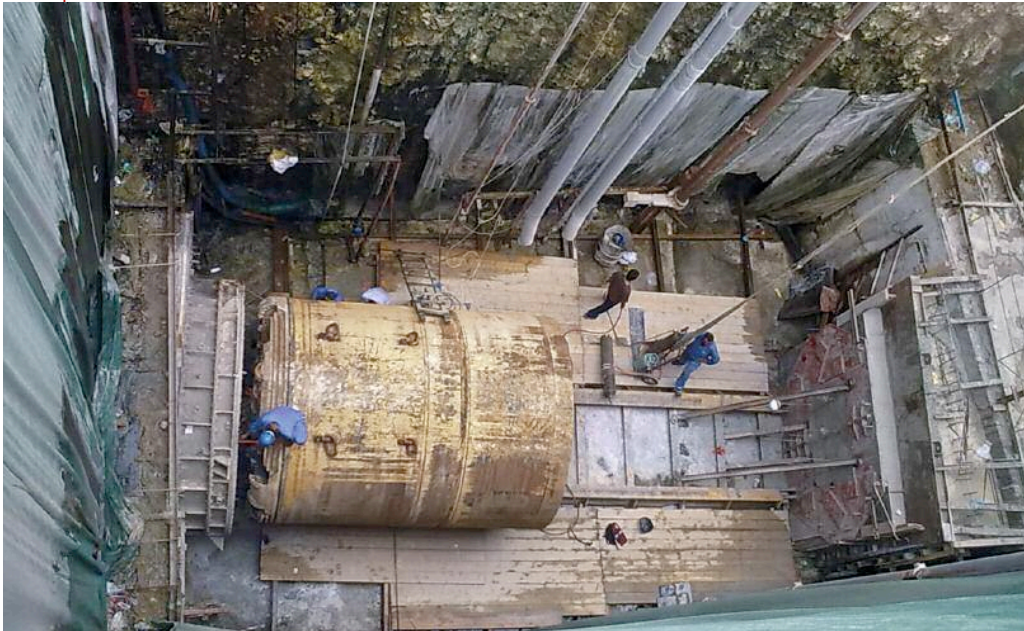
Left: Contractors are nearing the end of the storwater tunnel bore in Doha, Qatar
