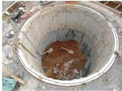
Above left: The terminal pumping station has a 37m diameter and is 40m deep Above right: A wall separates the dry well from the wet well
