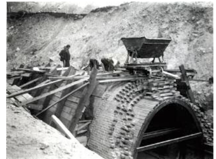
Above: The Victorian sewers are 130 years old
