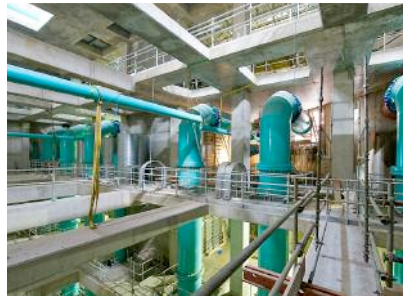
Above left: Six, 20t pumps sit in the TPS dry well
