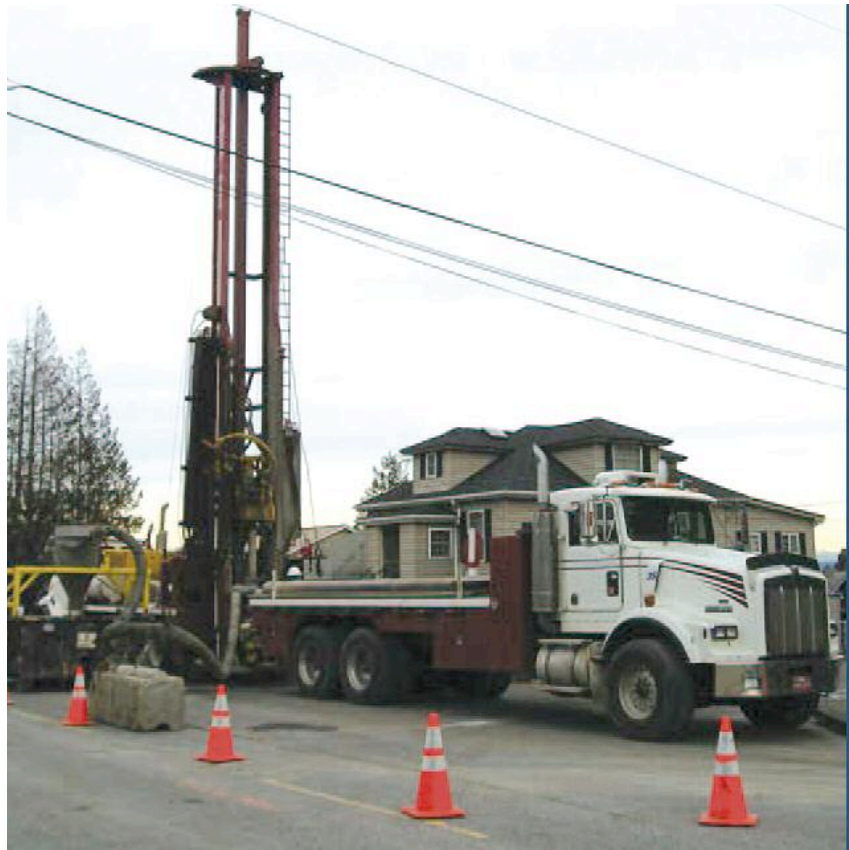
Above: Moretrench installation of dewatering wells at Beacon Hill with dual rotary drilling
