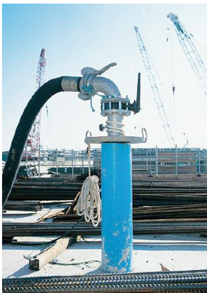
Above: Image 4 - A wellhead for deep well dewatering used on the Channel Tunnel Rail Link phase 2
