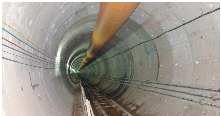
Below right: The Robbins EPBs are utilizing active articulation to avoid segment deformation in tunnel curves.
