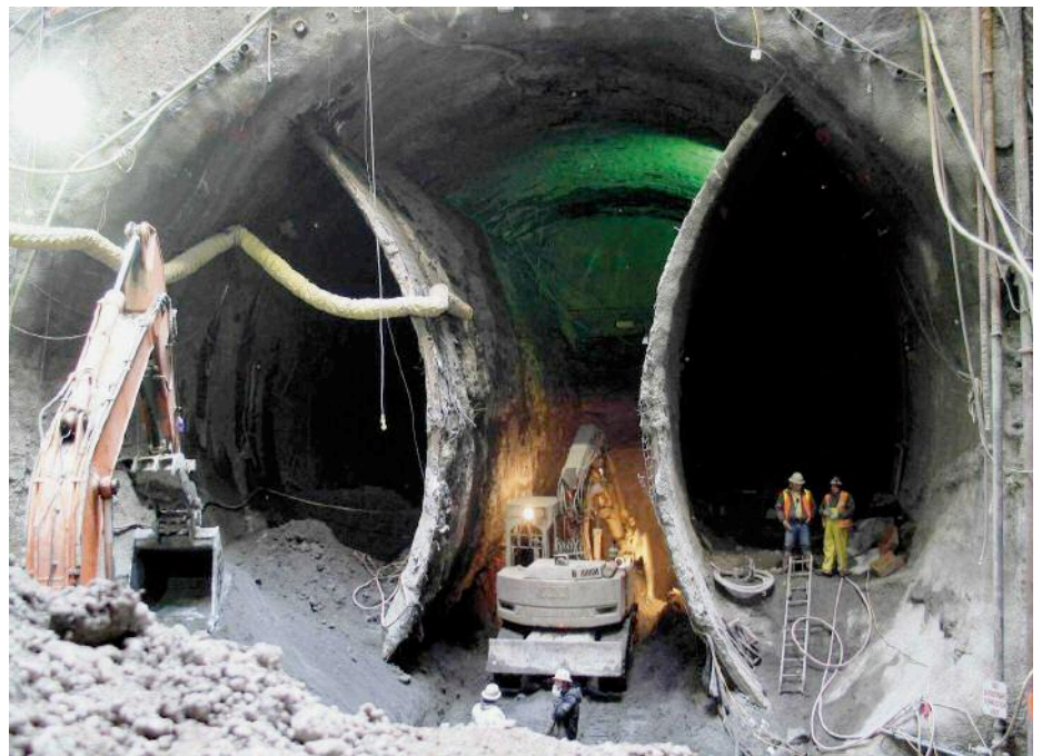
Above: Beacon Hill Station's concourse excavation with grouting pipes in the crown.
