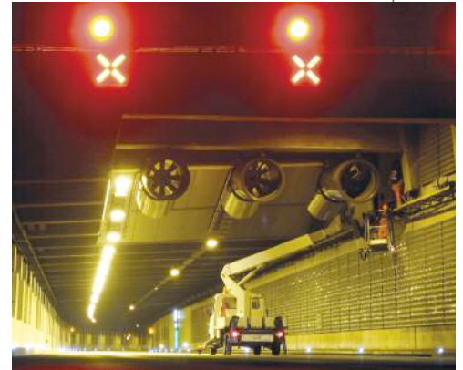
Above: New jet fans at the entry portal used installed during the refurbishment of the Schweizerhalle Tunnel on the A2 highway in Switzerland [Photo: HBI Haerter AG]
