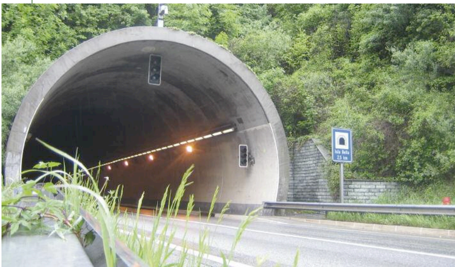
Below: Isla Bella Tunnel south portal before ventilation refurbishment [Photo: HBI Haerter]
