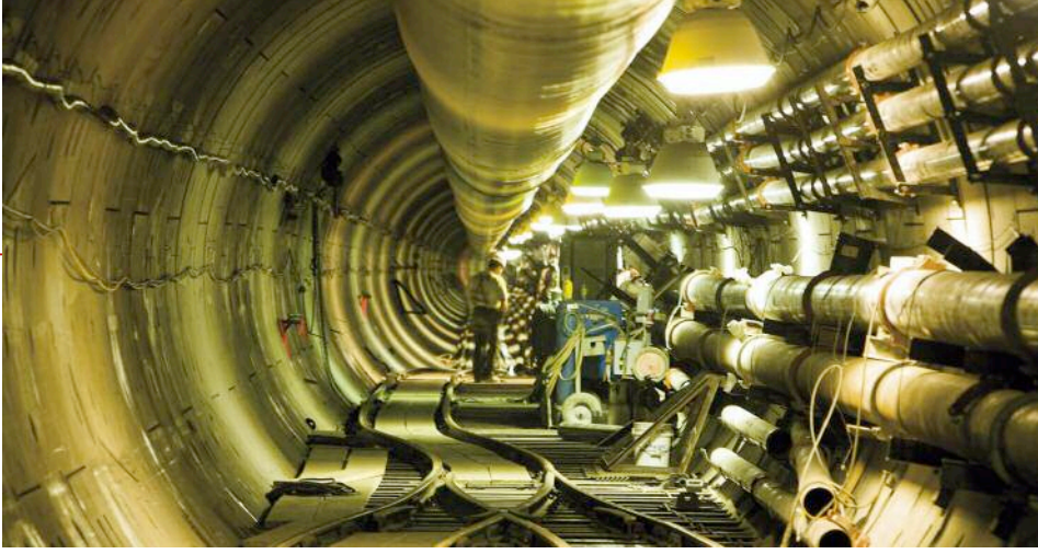
Left: Severe wear has shut down slurry machines on the Brightwater Conveyance Tunnel
