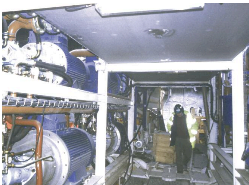
Above: Interior of the TBM, hydraulic pumps and overhead oil storage tank
