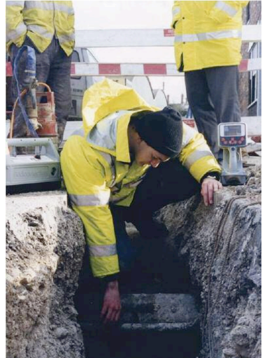
Above: A signal generator is attached to a utility for the location purposes. (picture courtesy of Infotec)
