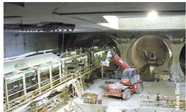
Above: Budapest metro Line 4-View of TBM south in Saint Gellert Station
