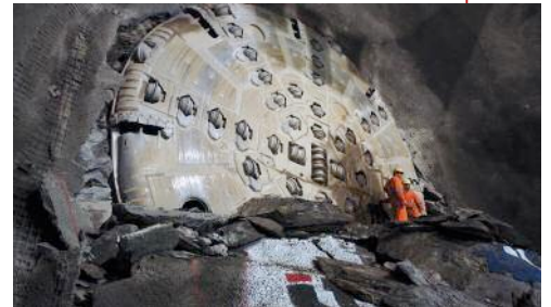
Below: The 9.7m Robbins TBM that recently completed a drive for the Ceneri Base Tunnel, in Switzerland
