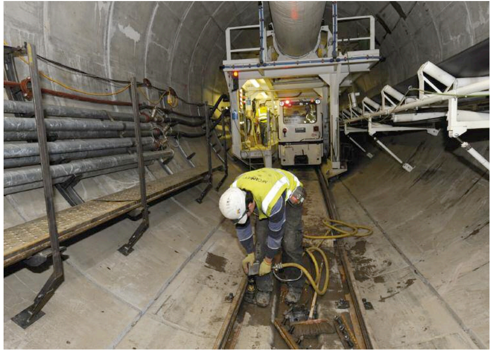
Above: Excavation at Heathrow airport for a tunnel that will be key to upgrading the baggage system
