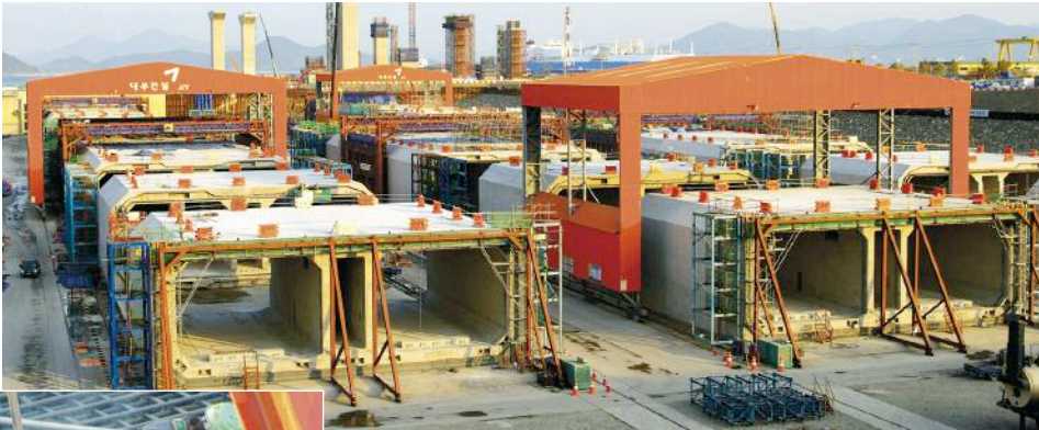
Right: Casting underway of sections to form immersed tube elements in South Korea
