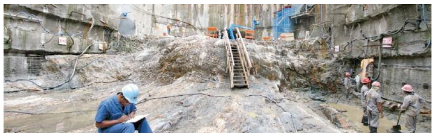
Below: Fig 4 - Mapping of the site, showing excavation changes in the bench height and final position of the lattice girders
