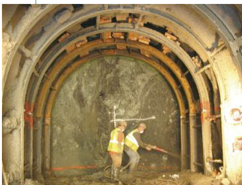
Top: Installation of spiling; Middle: Standing a steel set with the roadheader; Above: Application of shotcrete to blocked steel set
