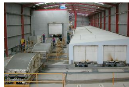
Above: Inside view of the concrete segment plant, with rolling moulds and water steam curing chamber
