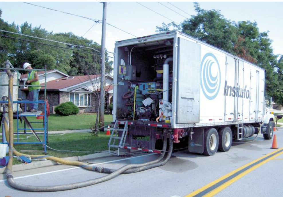
Above: A typical site set up on the Palos Hills rehabilitation project
