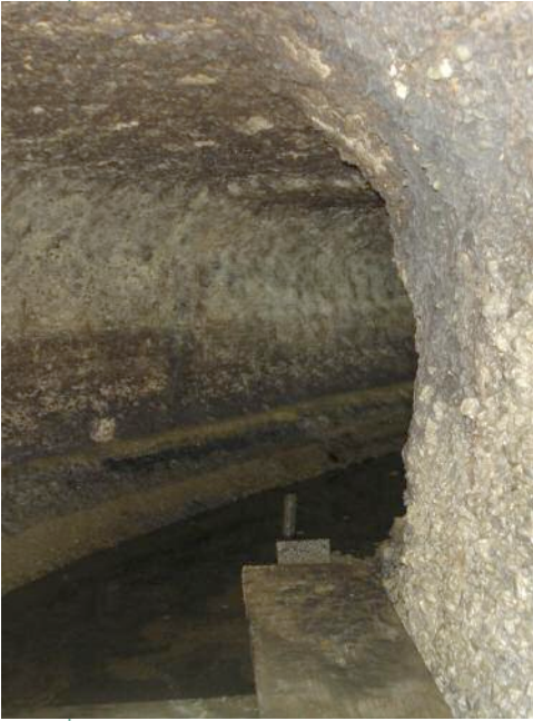
Above: The main drainage culvert condition prior to the GRP lining operation
