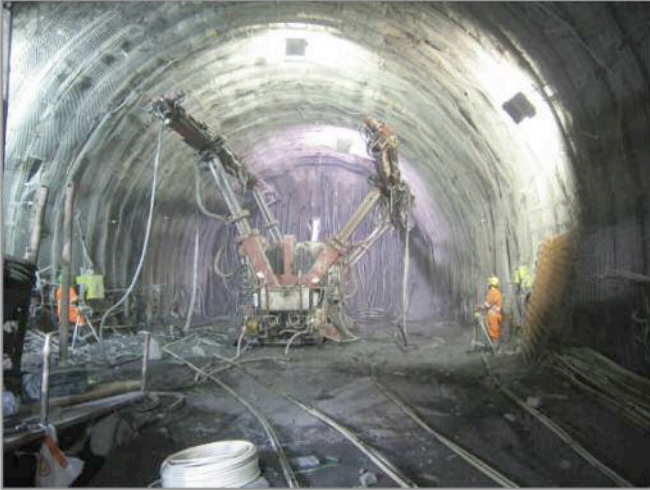
Lyon Turin Ferroviaire – Saint Martin La Porte, France Exploratory and service Tunnel Fiberglass nails
