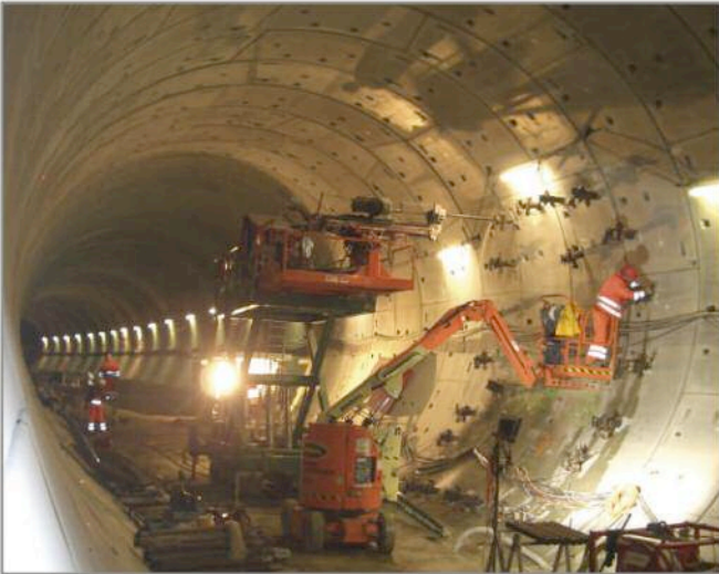
Hubertus Tunnel – Den Haag, Holland Highway Tunnel Ground freezing for construction of safety cross passages
