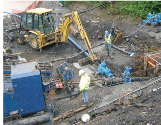
Above: Drilling into the Adit. Note the wellhead for pressure control of the mine water during the drilling operation
