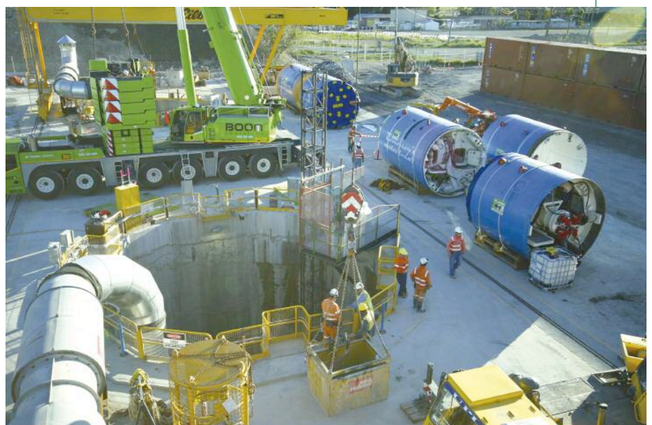
Right: A view of the sections of TIM on the surface waiting to be lowered down the 70m shafts
