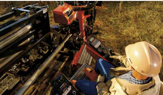
Above: Ditch Witch has recently upgraded both the Mach 1 and All Terrain versions of its well-established Jet Trac JT4020 HDD rigs
