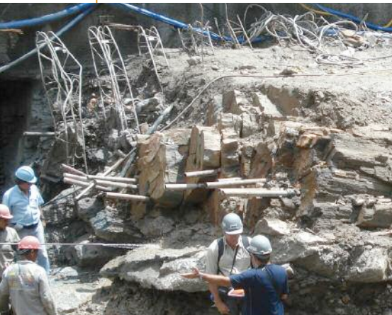
Above: Assessing the damage following the collapse, notice the bent lattice girders
