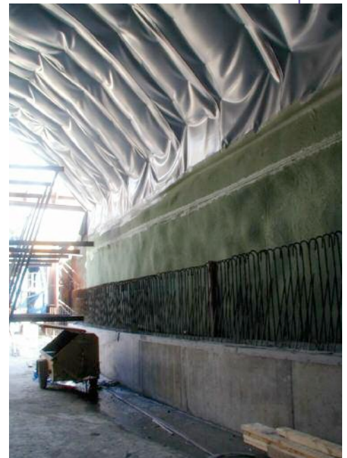
Above: Switzerland's Collombey tunnel, showing waterproofing membrane covering the crown and UGC's Masterseal sprayed on below groundwater level
