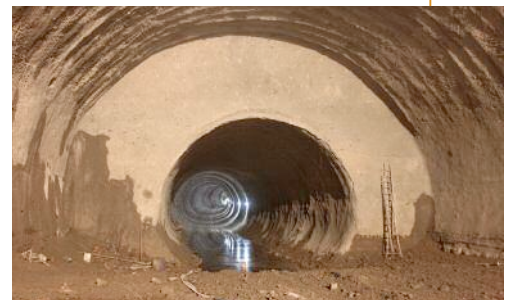
Top: A view of the heavy primary support in the top heading of the eastern station cavern. Lattice girders were at 0.85m c/c spacing, embedded in at least 35cm thickness of steel fibre-reinforced shotcrete
