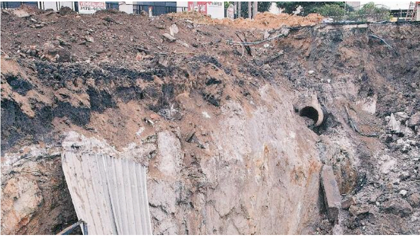
Above: Shear deformation on this major discontinuity when the cavern approached and passed below, may already have fractured this 700mm pipe
