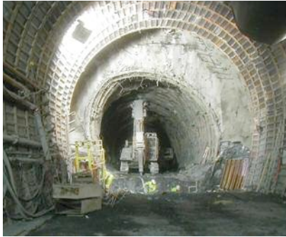
Above: View in the background of the support system initially adopted which underwent convergences up to 2m and later needed to be re-profiled
