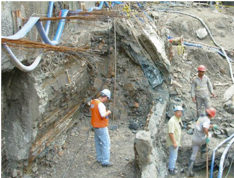
Above: Evidence for 'elephant-footing' failure
