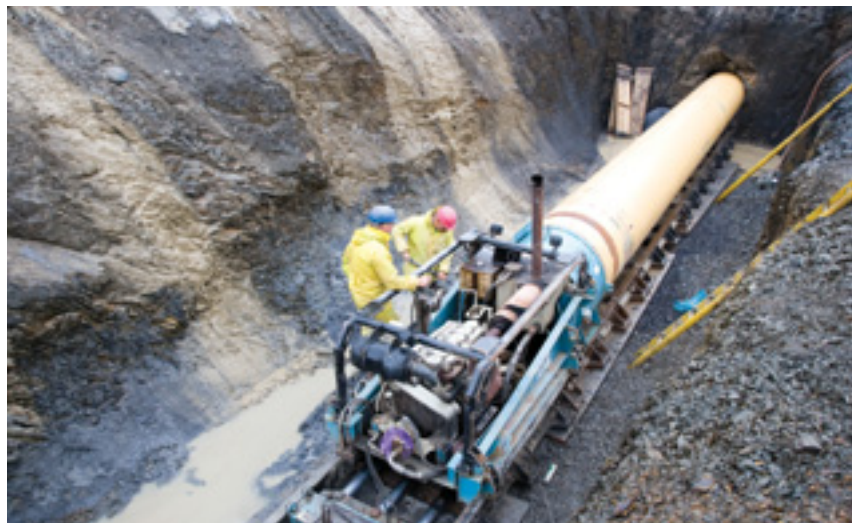
Above: The 20 hard rock crossings on Phase II of the Milford Haven Gas Connection Project utilised three Robbins SBU-As
