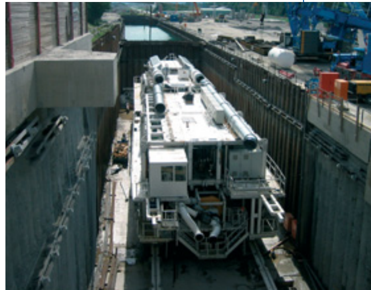
Right: Assembly of the Herrenknecht Mixshield for the Jenbach Tunnel ahead of a cell of subaqueous open-cut work
