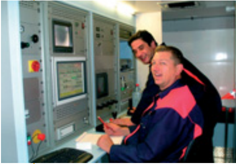
Above: The control console onboard the UV lining truck
