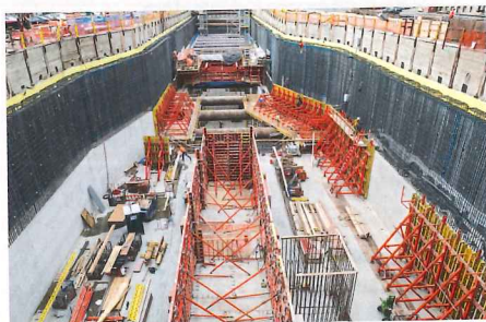
The formwork solution is based on system components of the VARIOKIT engineering construction kit. The traveler system for the bottom level is also used in the upper levels.
