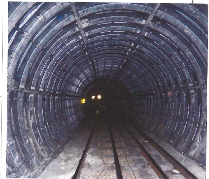
Above and bottom right: Other recent work on the London Underground includes re-lining a section of the Jubilee Line
