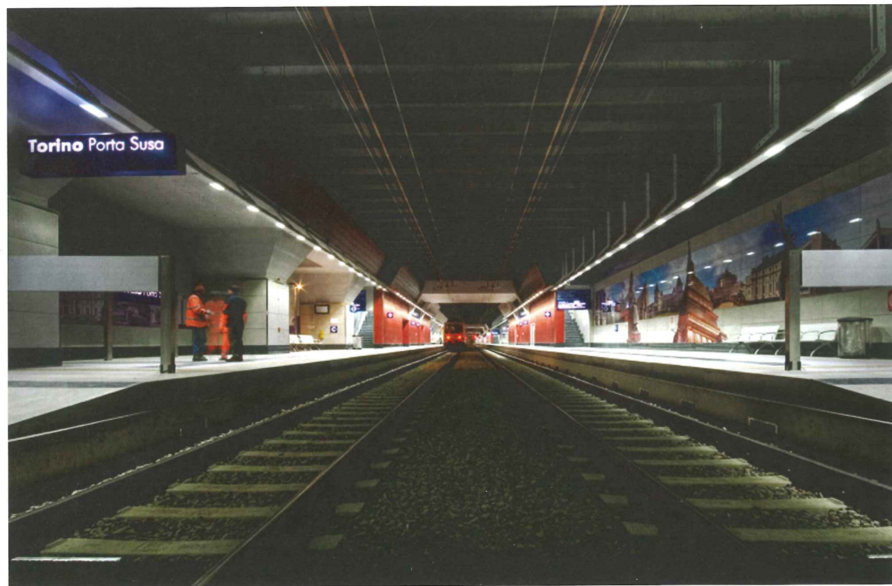
Below: Full LED lighting solution for metro station in Turin
