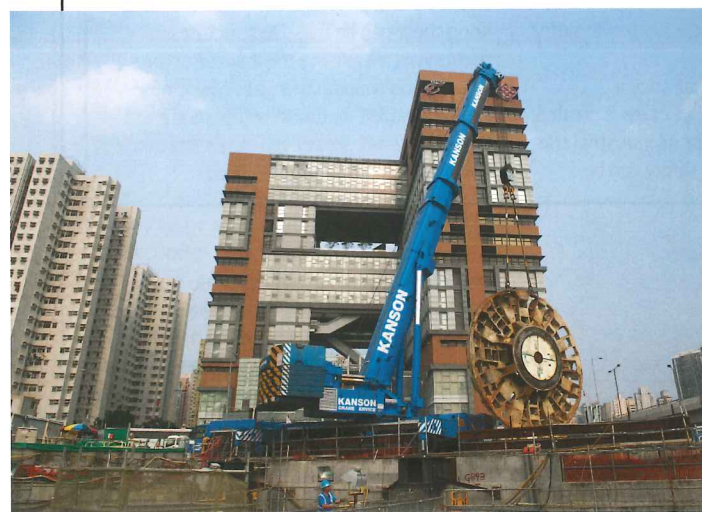
Below: XRL Contract 820, Mei Lai Road to Hoi Ting Tunnels, Hong Kong © Arup
