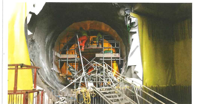
Top: The caisson shaft, from which the majority of tunnelling work was executed
