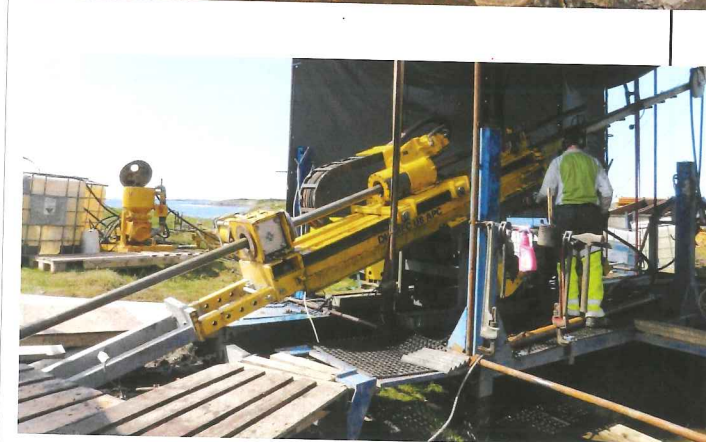
Top: Challenges in volcanic geology: Progressive collapse during excavation Vadlaheidi road tunnel, Iceland PHOTO BJORN HARDARSON (GEOTEK)
