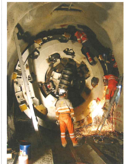
Right: Marti Tunnelbau AG's 4.4m diameter TBM has been used on 9.7km of tunnel since its use on the Bracons tunnel (pictured) in 2006, and on 12.3km of tunnel since its original manufacture in 2001
