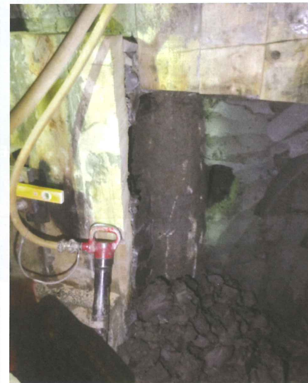
Left: Figure 15, The pile was initially left in place, to ensure checks could be conducted on its provenance; the face was timbered at this point to ensure personnel were not exposed to potential wedge/block failures
