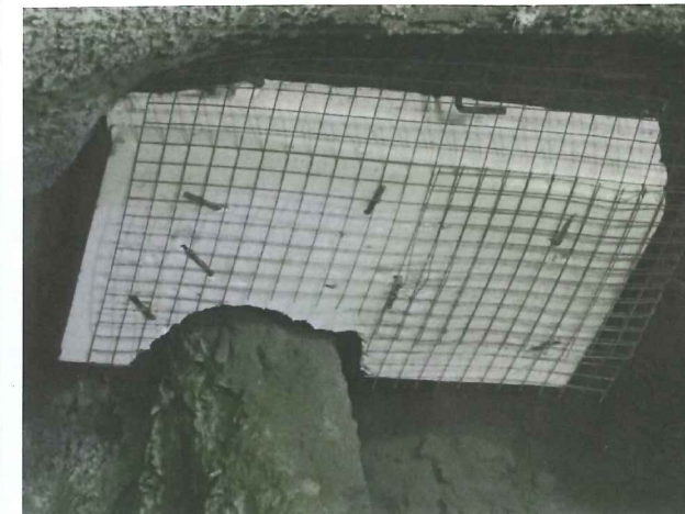
Left: Figure 14, Physical Separation applied at C300/C410 (BFK), incorporating a steel mesh
