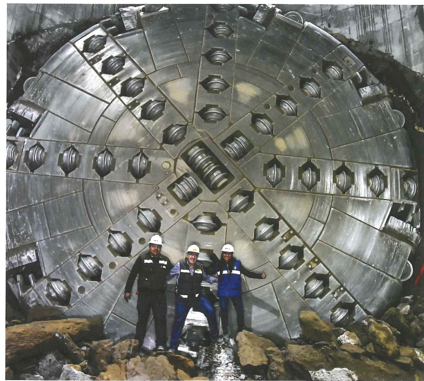
Top: Personnel from the manufacturer pose after breakthrough Above: After celebrations, the contractor will construct the secondary lining
