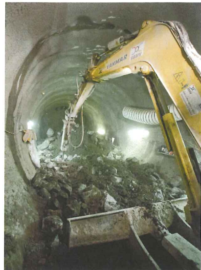
Left and Below: Work at Finsbury Circus in January 2013; and the grout shaft earlier, in February 2012
