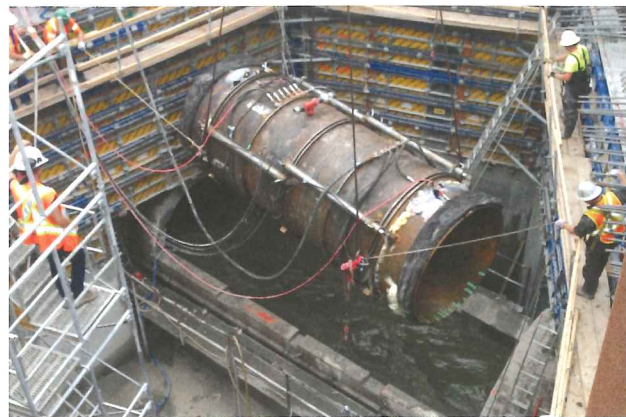
Above: YDSS flume bypass retracted and lowered
