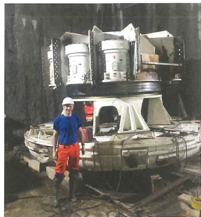
Left: The Robbins machine was launched to bore the final 9km of tunnel in summer 2016
