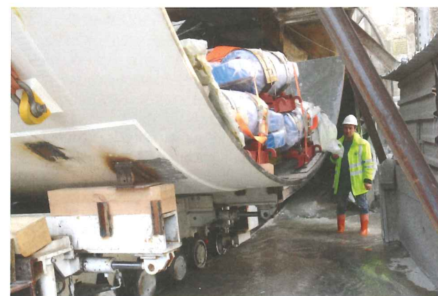
Right: Specialised transport cars with hydraulic lifts were used to transport some of the TBM components through the tunnel and into the launch chamber
