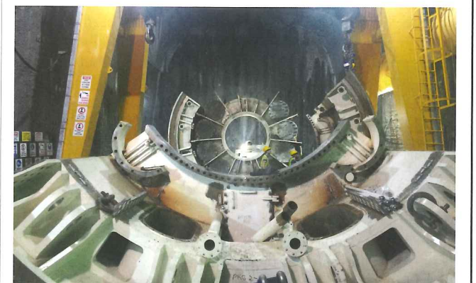
Below: The Robbins Crossover machine was assembled several kilometres inside the tunnel in an underground launch chamber
