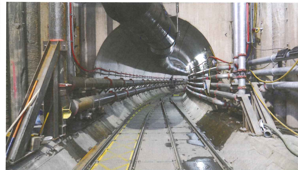
Top: A view of one of the bifurcation shafts that link the tunnel to the existing network Above: Looking through the portal of the new Shieldhall tunnel
