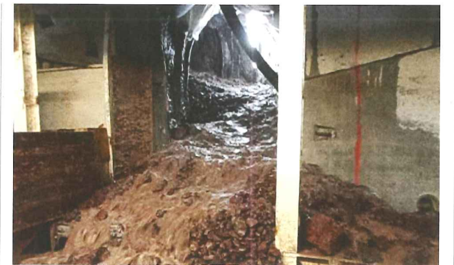
Above: Two double shield TBMs became irretrievable stuck or damaged amid massive mud and water inflows
