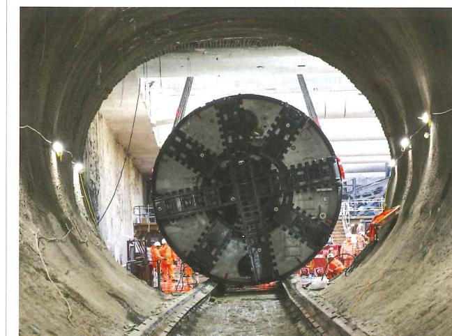
Below: The new tunnel diameter is 5.2m, and existing tunnel diameter is 3.8m
