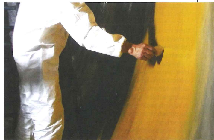
Right: Wet film dipping to measure the thickness of the first layer of Integritank HF on Line B of the Buenos Aires metro in Argentina
