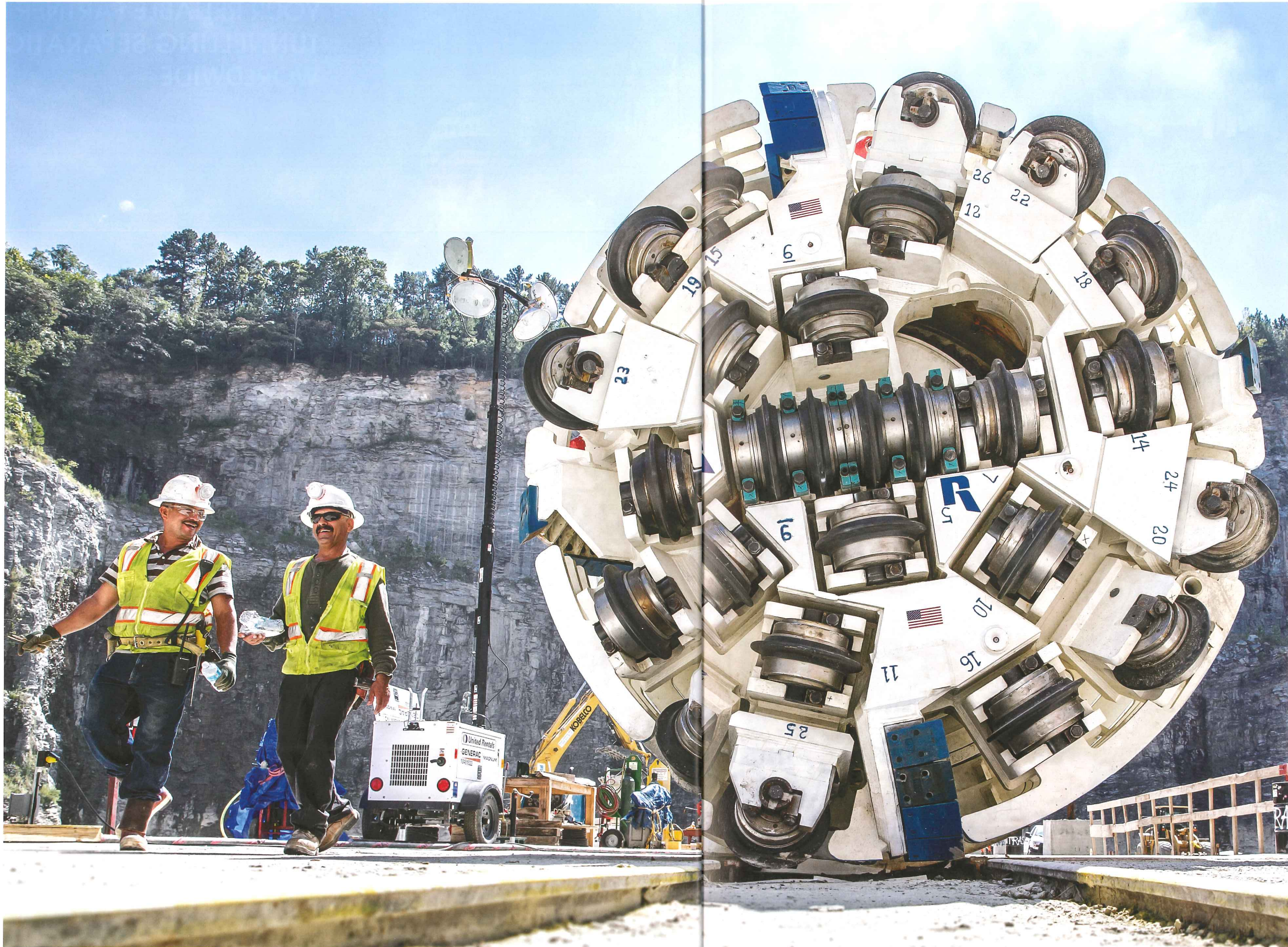
Left: The 3.8 m diameter Robbins Main Beam TBM is now boring the 8km Bellwood Tunnel in Atlanta, Georgia, USA after being walked forward 30m into a starter tunnel. The Bellwood The alignment runs from an inactive quarry and run below a water treatment plant and reservoir before ending next to the Chatta-hoochee River. The project is an emergency water supply tunnel being bored through granite
