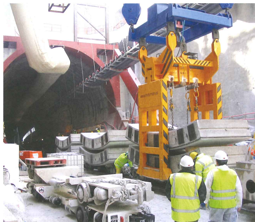
Top: Cast-in gaskets typically have a neater finish than glued methods Above: Segments fitted with cast-in gaskets heading to the face
