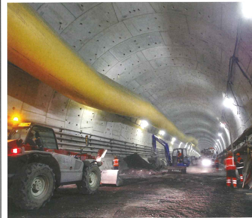
Top: Segments bound for a metro tunnel in St Petersburg Above: Construction of the Green Heart Tunnel, Netherlands
