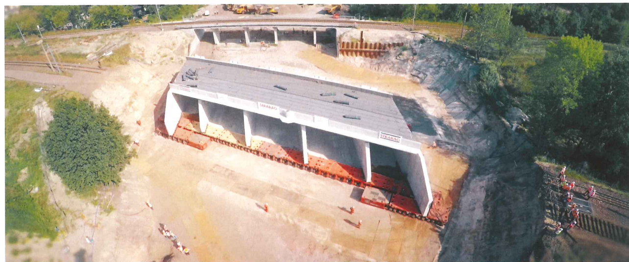
The prefabricated section is moved into place by 104 axle lines of Self Propelled Modular Transporters
