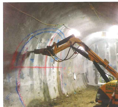
Left: Commencement of breakout using a hydraulic breaker at Crossrail's Farringdon Station
