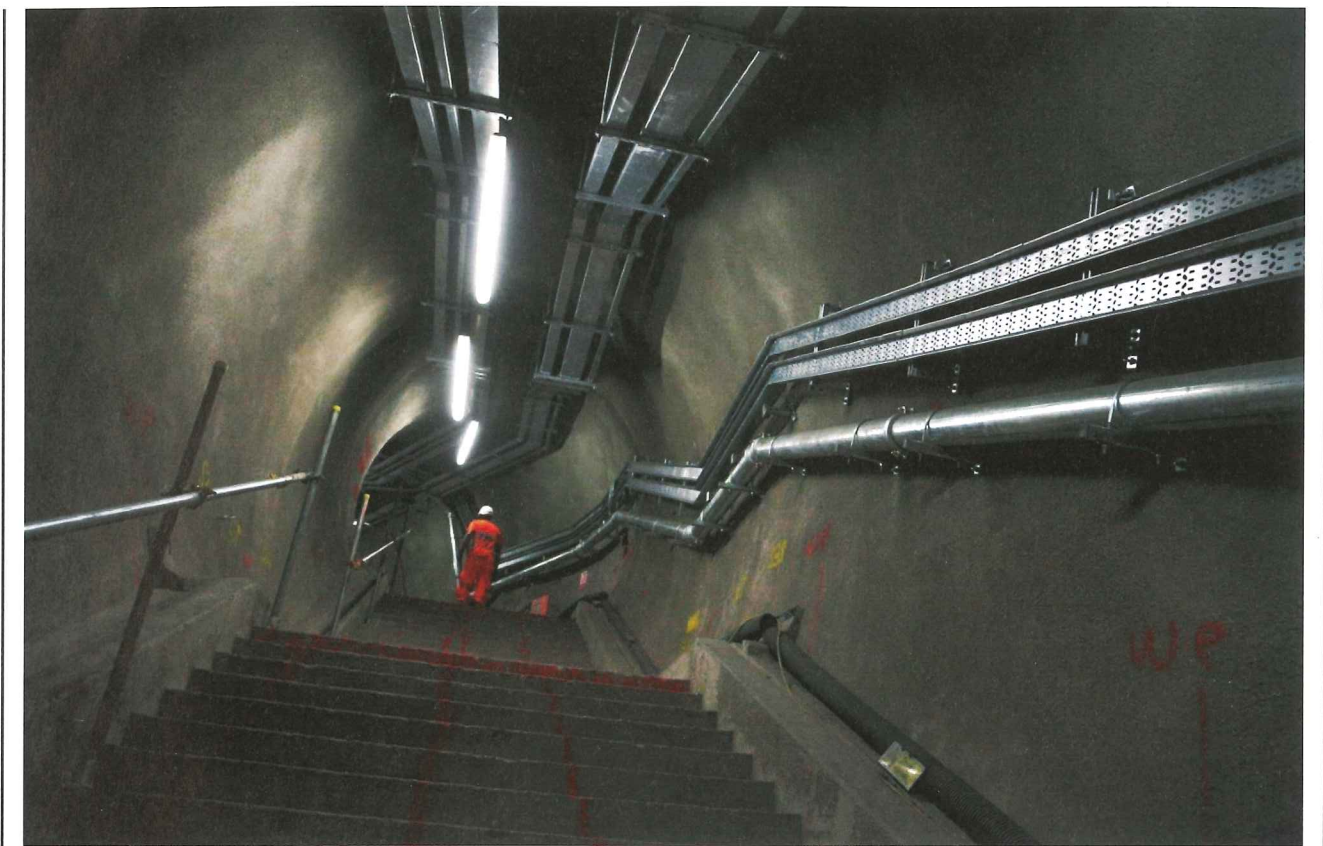
Above: A new SCL tunnel proving access to the Jubilee Line platform
