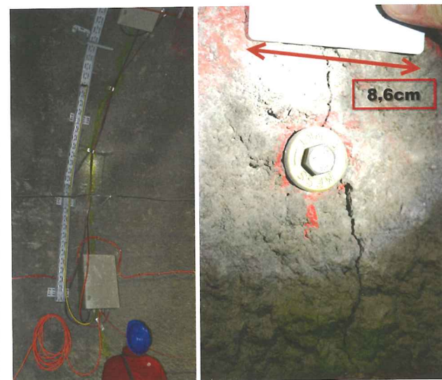
Above: Figure 6, Observed crack and high internal forces in the model
