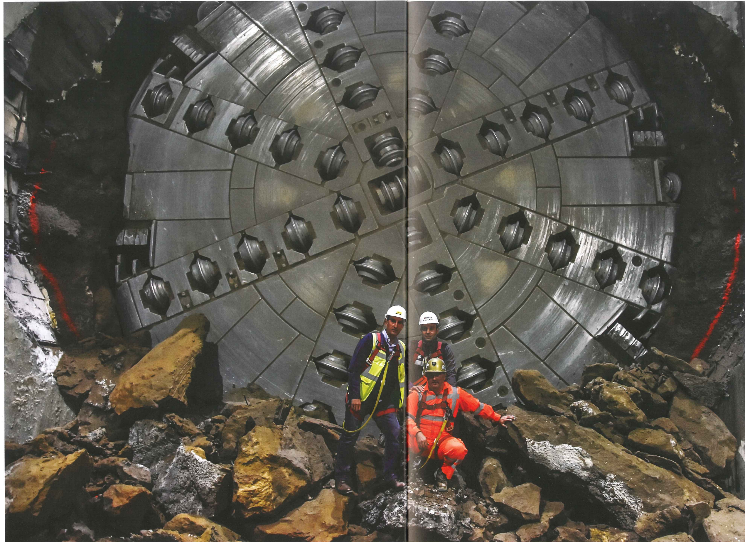
Left: Break through on the Túnel Emisor Poniente (TEP II) project in Mexico
