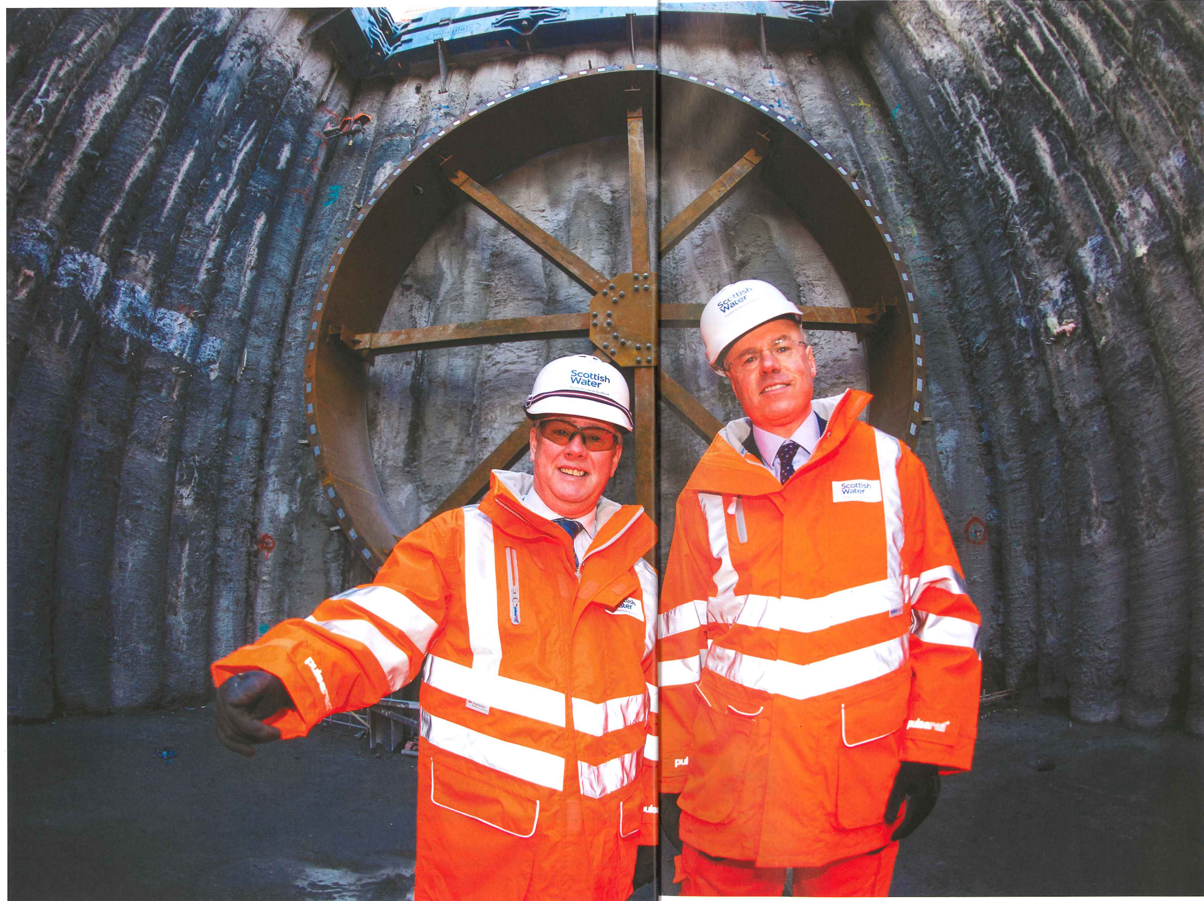
Left: Scottish politician Keith Brown, who has responsibility for infrastructure, investment and cities in the devolved parliament, recently visited the Shieldhall Tunnel project in Glasgow. The GBP 100M sewer project will run for 5km and will be 4.7m in diameter. The first 250m of the tunnel, and the launching chamber, are open cut. The main bore is being driven by TBM
