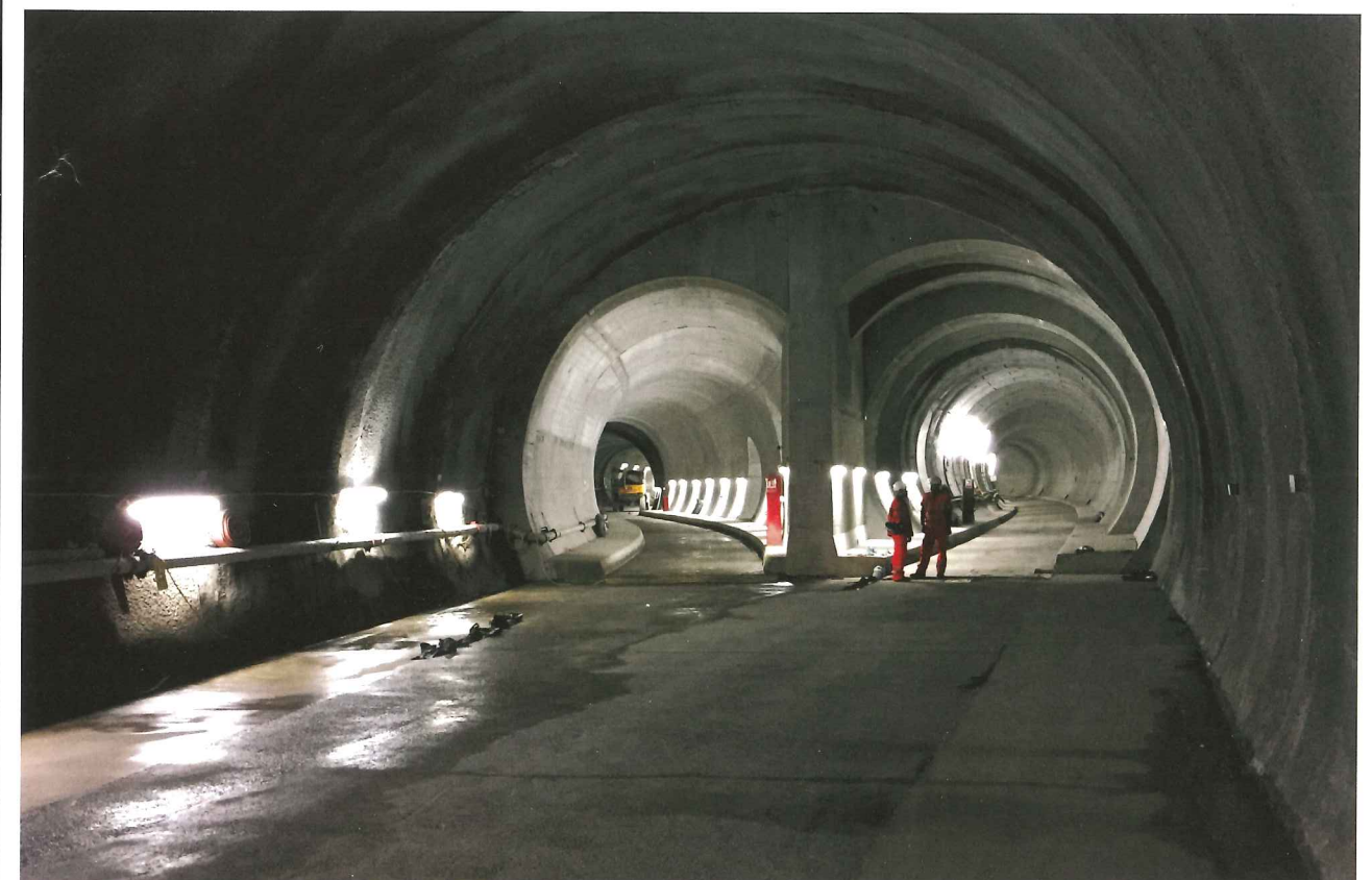
Below: Work at Fisher Street took place under one of the most congested areas in London
