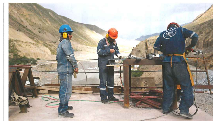
Above and Below: The Cheves power plant is the first greenfield project developed and constructed by Statkraft alone in South America.
