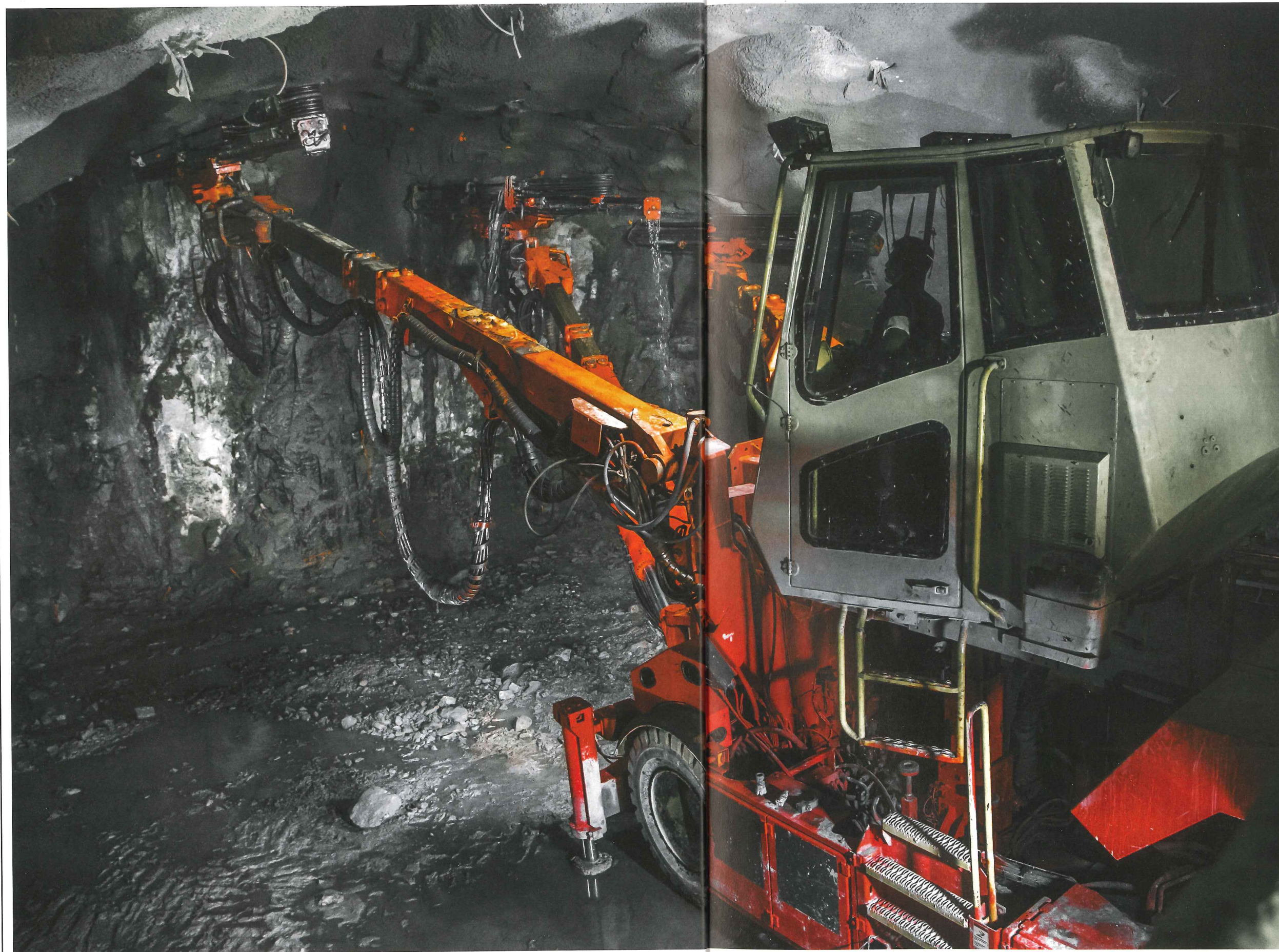
Left: Sandvik DT1131-SC jumbo in operation at the Cumbres de Llano Largo Mountain tunnel in Mexico. The 3.2km-long drive should be finished in July for a cost of USD 213M. It will be the longest road tunnel in the country. The maximum excavation area achievable by the equipment is 18m across by 11m high
