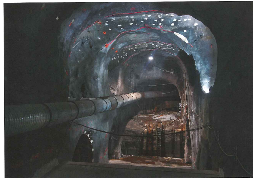
Early cavern work on MTA's East Side Access project This photo shows work on going in October 2013. PHOTO: METROPOLITAN TRANSPORTATION AUTHORITY / PATRICK CASHIN
