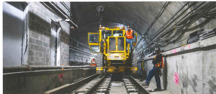
First work train traverses the Second Avenue Subway line in New York, USA
