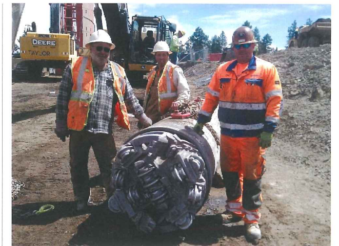
Above: Crew members from Stadel and Robbins were able to hole through on line and grade after achieving up to 50 ft (15 m) of advance per day
