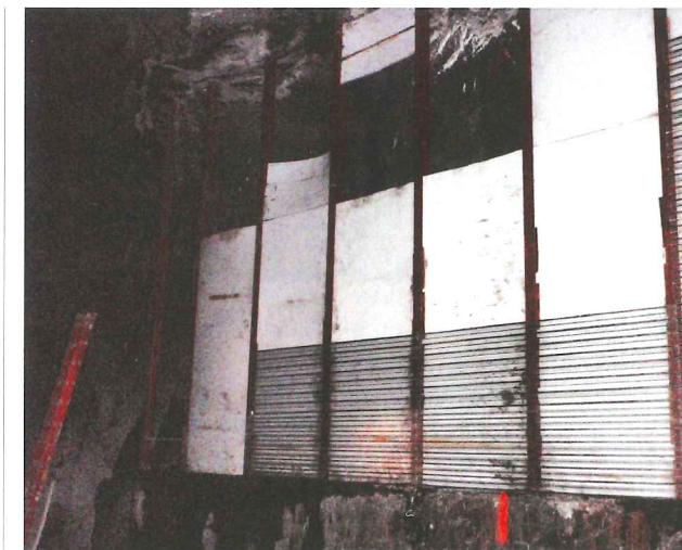
Above: Figure 7. Deterioration of Allegheny Tunnel ice shields and supports
