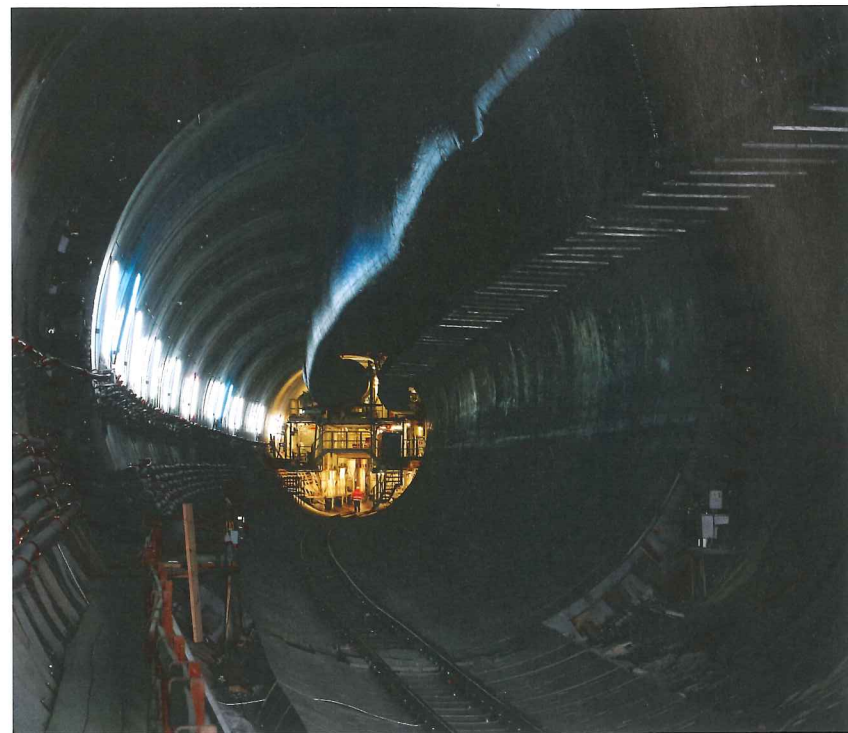
Above: View of the excavation face (left) and rear of the shield
