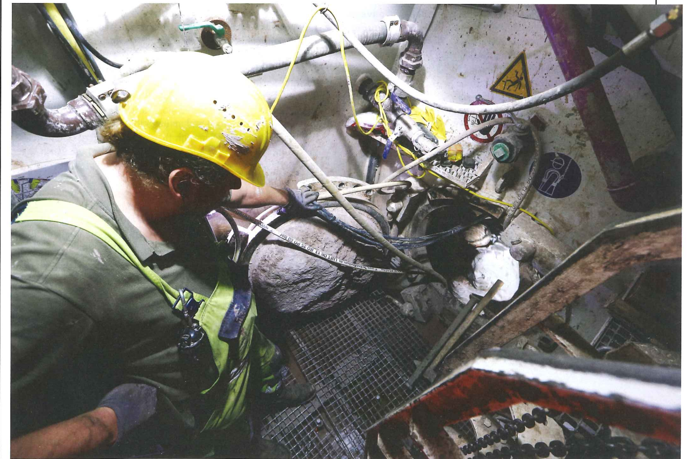
Below: As Tunnels and Tunnelling went to press, the Herrenknecht machine was soon to undertake a planned stop
