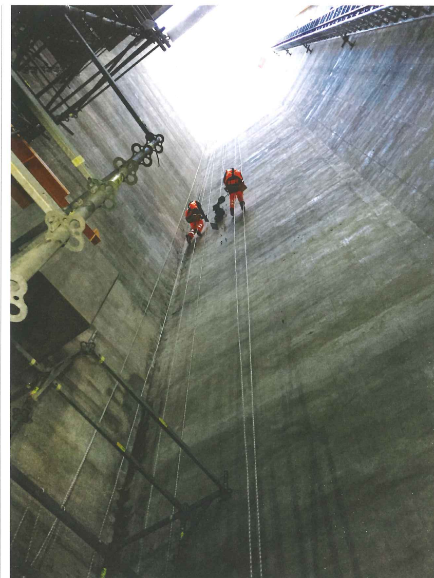
Above: Workers equipped with climbing gear install ventilation on a Lee Tunnel shaft
