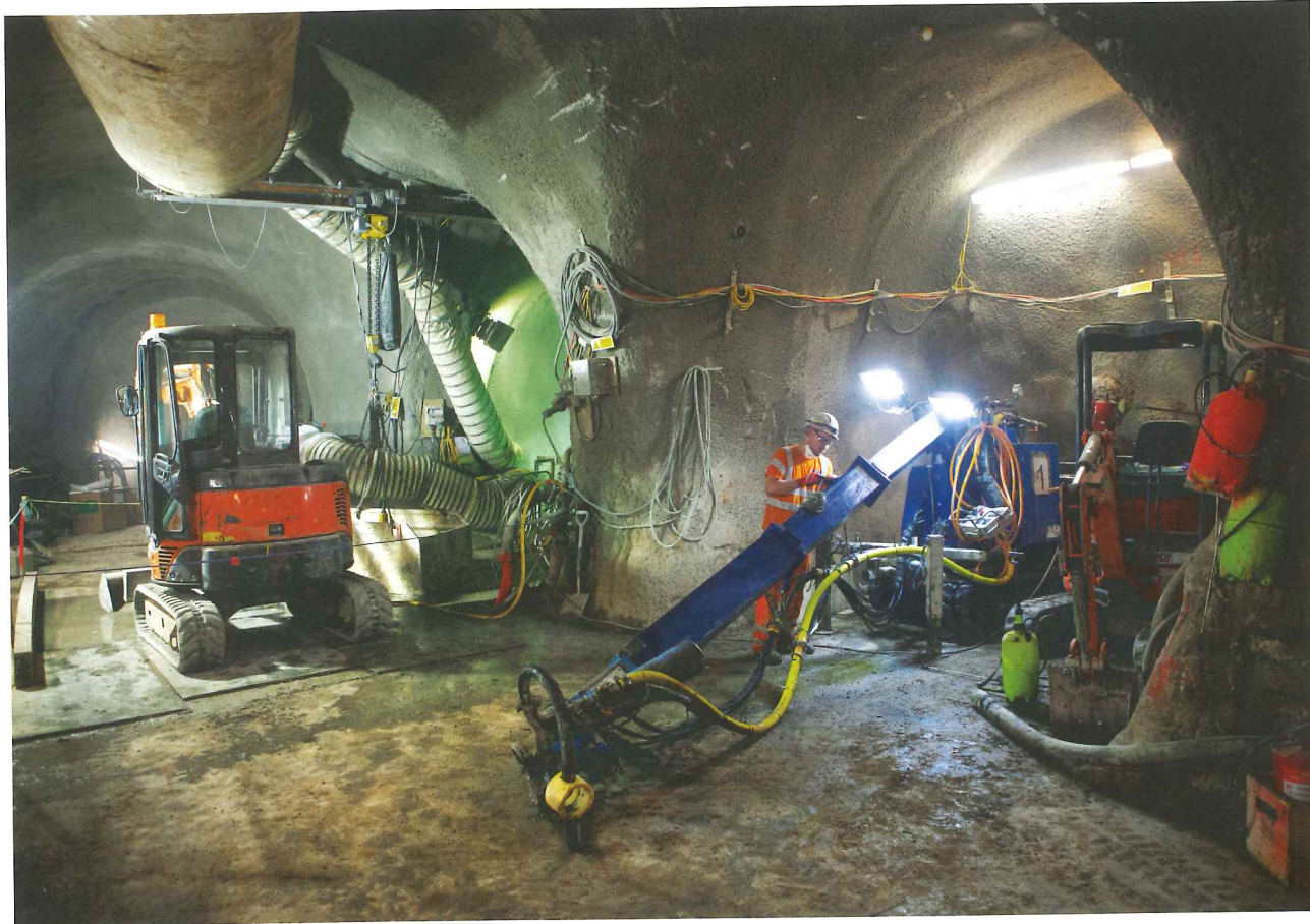
Above: Specialist plant for forming the SCL tunnels shown in the interchange passages
