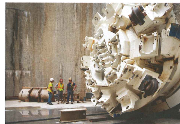
The 3.96m-diameter Main Beam TBM being used to bore Hawaii's longest tunnel
