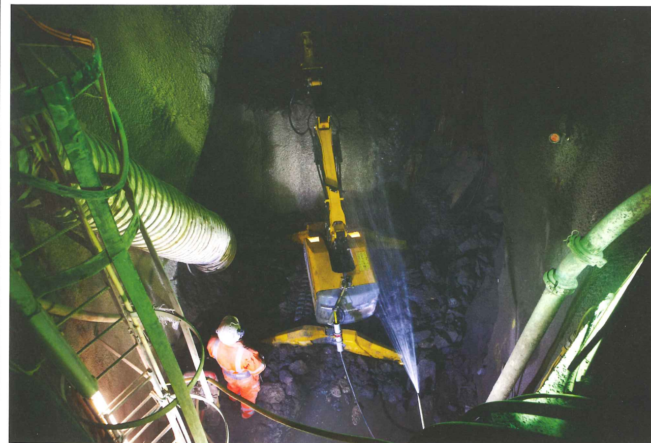
Below: Digging the new SCL tunnel leading to the Jubilee line platforms viewed from the new lift shaft
