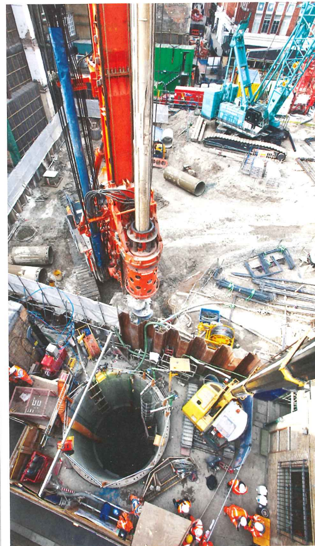
Right: Aerial view of one of the 13 shafts required for grouting this 2km section of Crossrail
