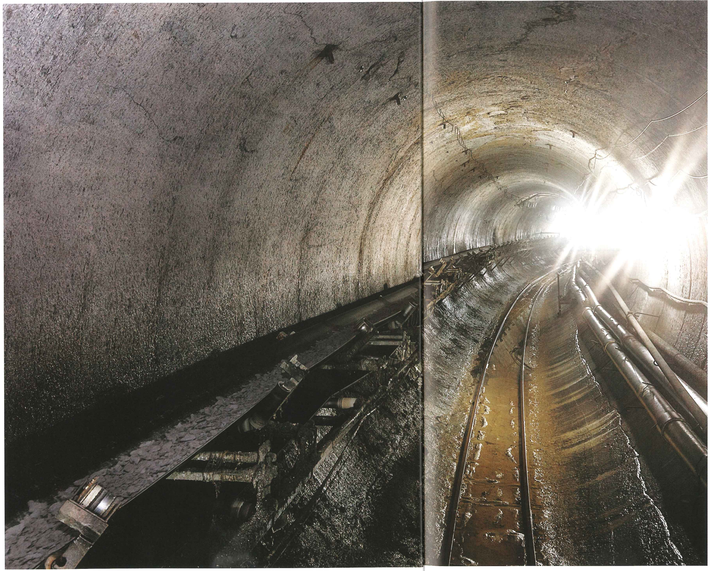
Left: On March 5 a Robbins 6.2m-diameter TBM finished boring a 2.8km-long extension tunnel, known as the Eagle Creek Tunnel, for the Indianapolis Deep Tunnel System in Indiana. The contractor is a joint venture of Shea and Kiewit.
