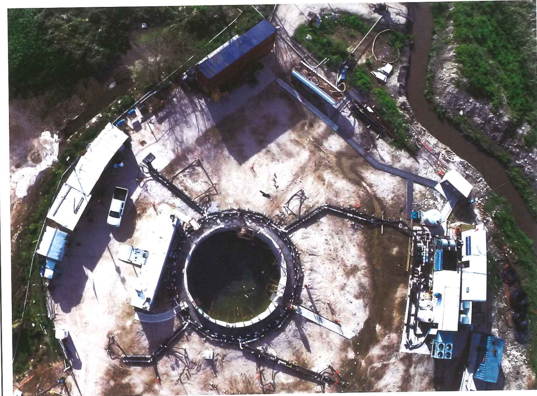
Left: Aerial view of Access Shaft Three at the Sistema de Potabilizacion Area Norte project in Buenos Aires, Argentina. See page 40
