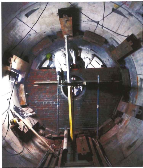
Left: 1.5m thick brick bulkheads were constructed in the tunnel to prevent material inflow in case of shaft failure
