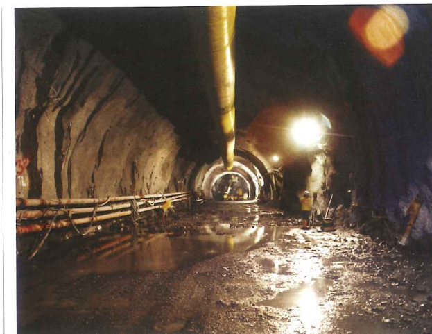
Above: Colombia is considered to be a pioneer of tunnel work in Latin America
