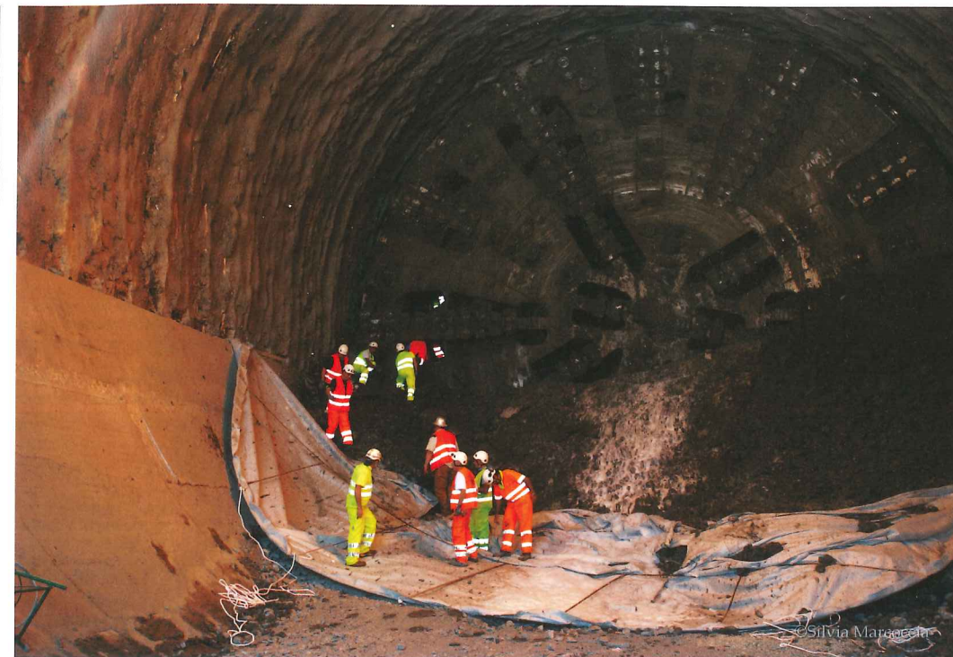
Left: TBM breakthrough on Italy's Sparvo Tunnel project. This machine was previously the largest diameter EPBM. Page 31
