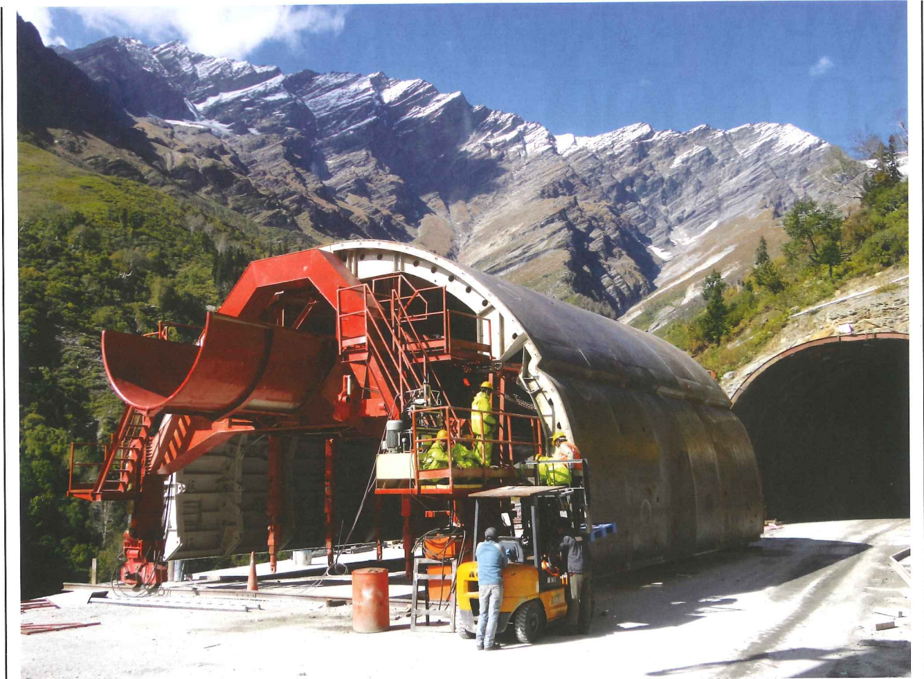
Above: Formwork for cast in-situ lining at the Rohtang Tunnel project in India
