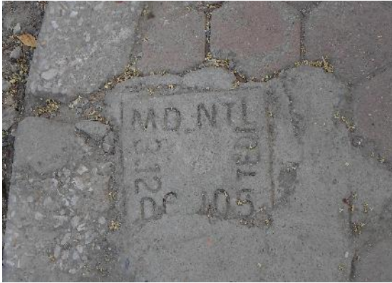
DC-105 (Hỏng nôm sứ/Damaged)
